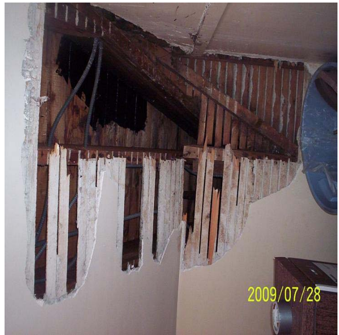
402 Essex St., 2nd Floor – Hole in Wall
