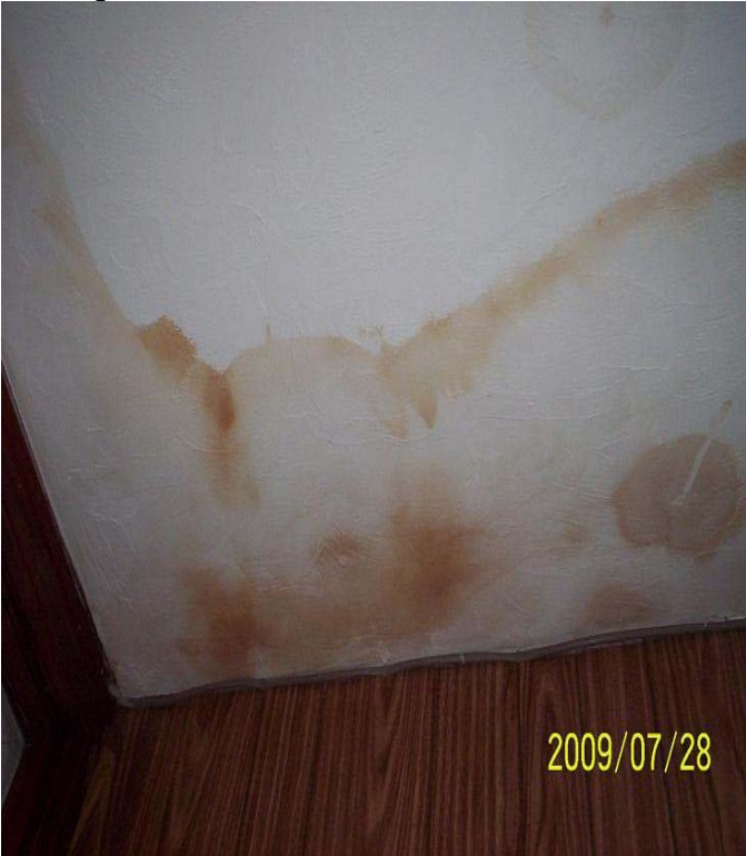
Peeling Paint, and Water Leak
