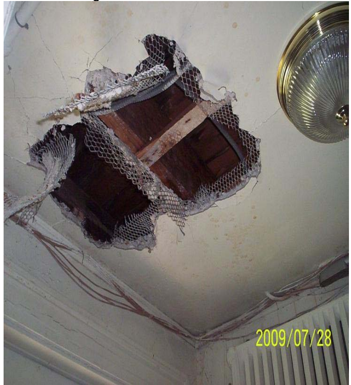
Hole in Ceiling
