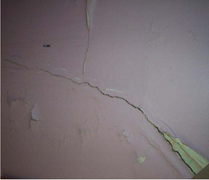
Conference Room: Peeling Paint and Cracked Walls
