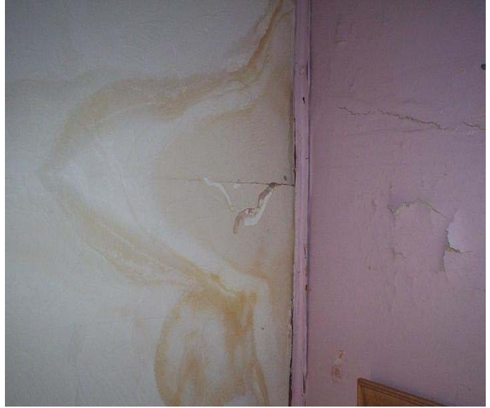
Conference Room: Peeling Paint, Cracked Walls, and Water Leak
