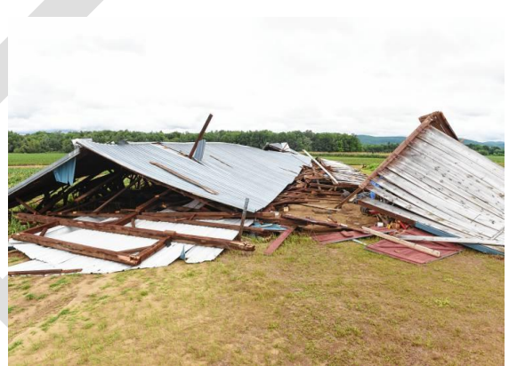
A microburst in June 2020 downed crops and pine trees on one farm in Whately, and damaged a tobacco barn and farm equipment on another farm. Concerns about the increasing intensity of wind events was discussed during the CRB workshop. Photos courtesy of the Greenfield Recorder.
