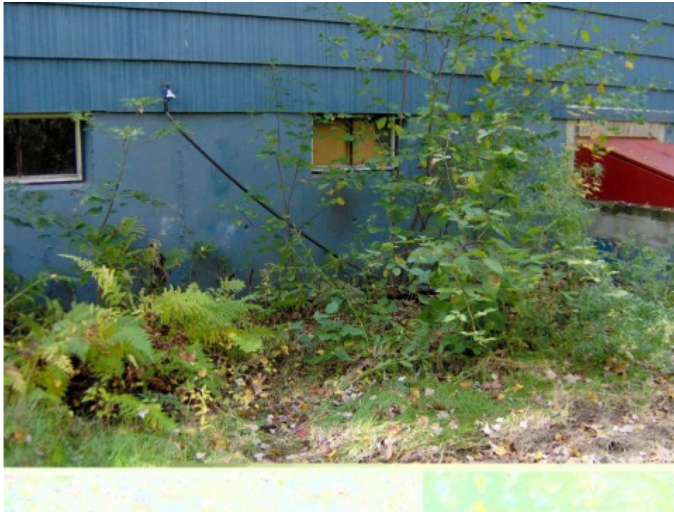
705-C Development 43 North Street Window Missing
