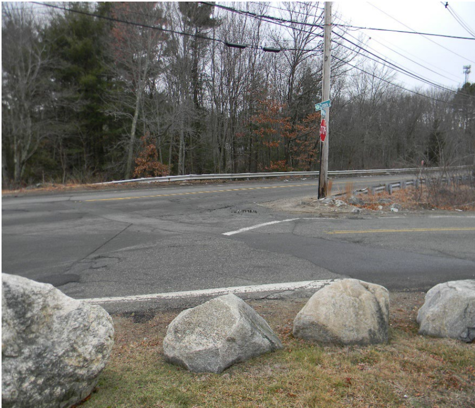
Substandard roadway geometry
