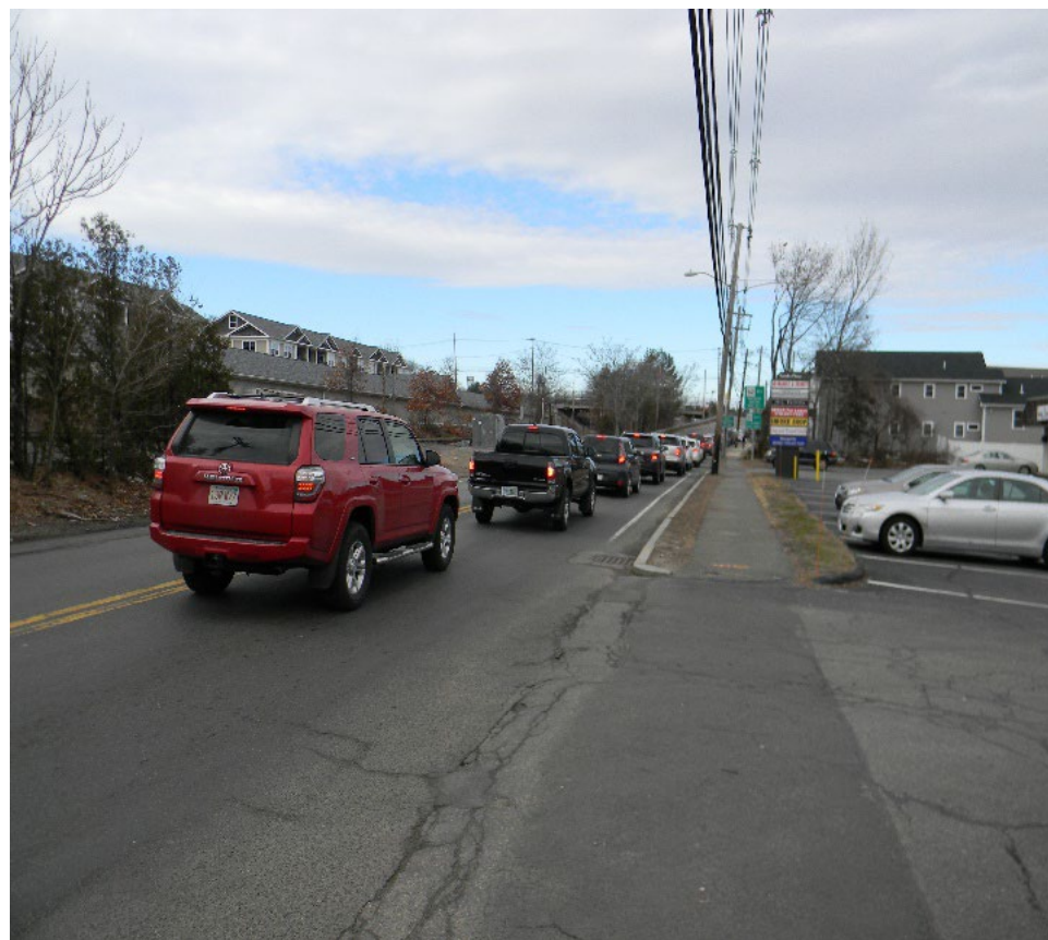
Existing Conditions: Poor pedestrian accommodations, and limited sight distance. Site of frequent vehicle crashes.
