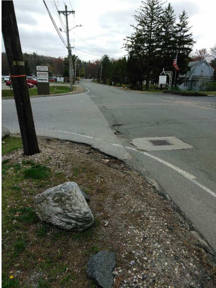
Limited/deficient drainage and poor pavement conditions
