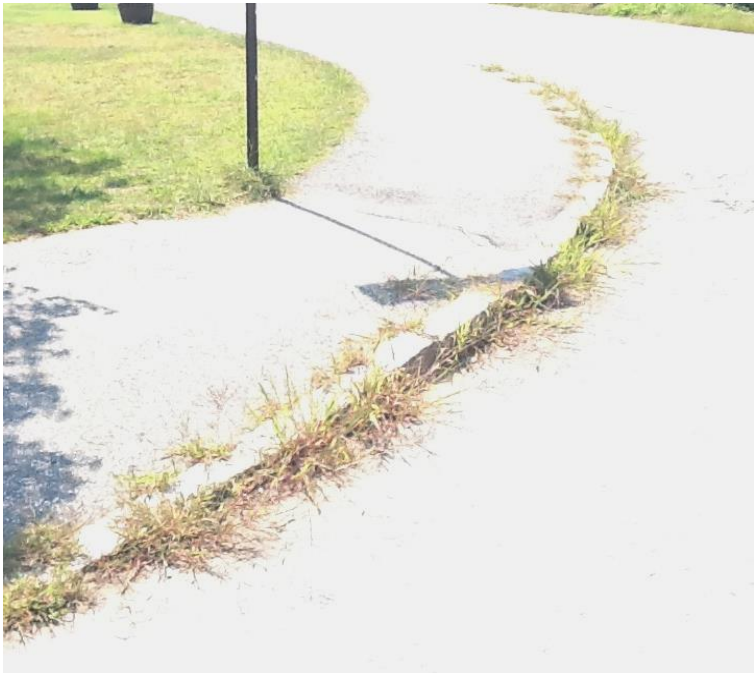
Figure 2 – Detrimental Vegetation at Cherokee Lane Subdivision Detrimental grass damages Town infrastructure and is unsightly.
