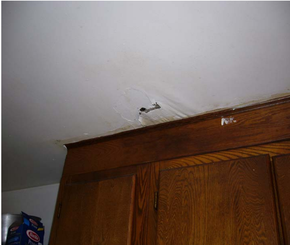
200-1 Development, 83 Creston Avenue – Kitchen Ceiling has Hole
