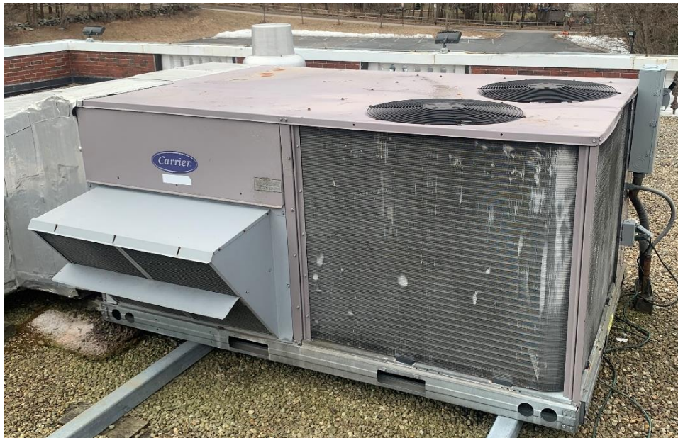
Photo 1 – Rooftop Air Handler RTU-1
