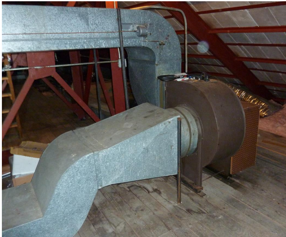
Photo 1 – Representative Exhaust Fan
