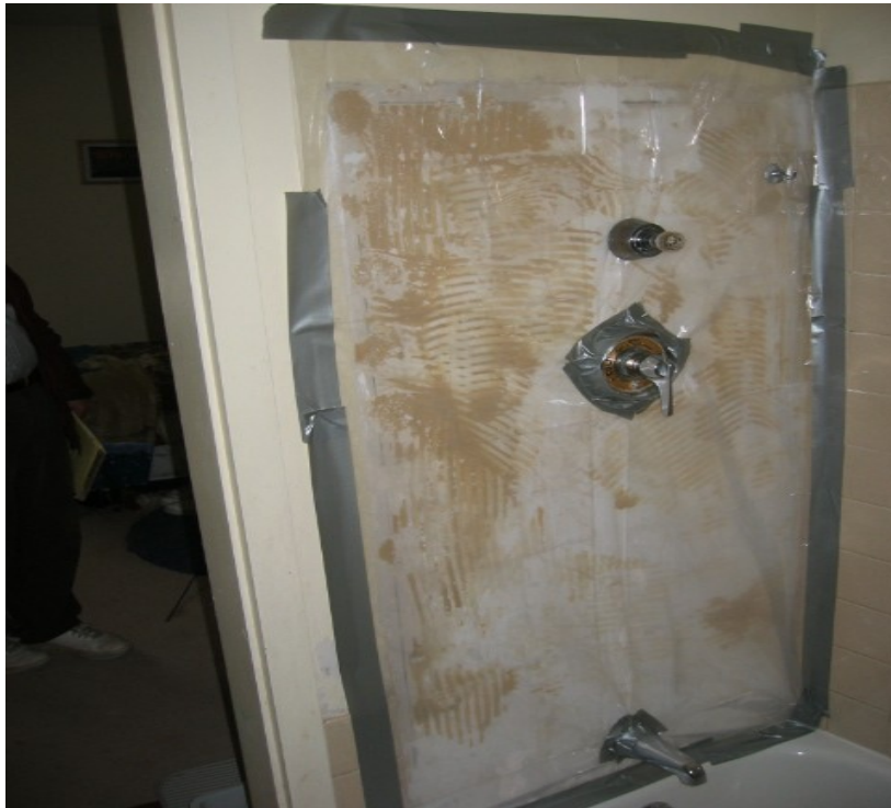
667-1 Development, Long Pond Plaza, Unit #8 Bathroom – Shower Stall Tiles Missing, Wall is Covered with Plastic Sheeting and Tape
