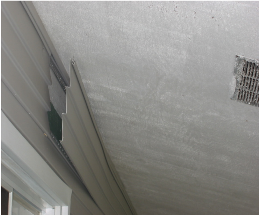
667-1 Development, Long Pond Plaza Siding is Lifting Off the Building
