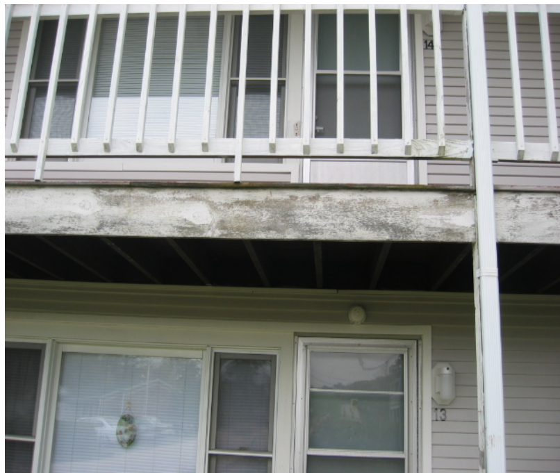
667-1 Development, Long Pond Plaza Mold on Balcony Wood
