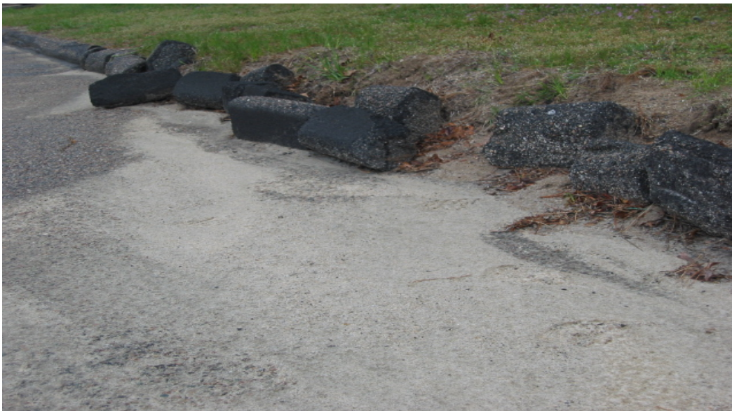
667-1 Development, Long Pond Plaza Damaged Berms on Long Pond Plaza Road
