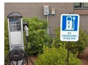
The new electric vehicle charging station outside the Lasry Center for Biosciences.
