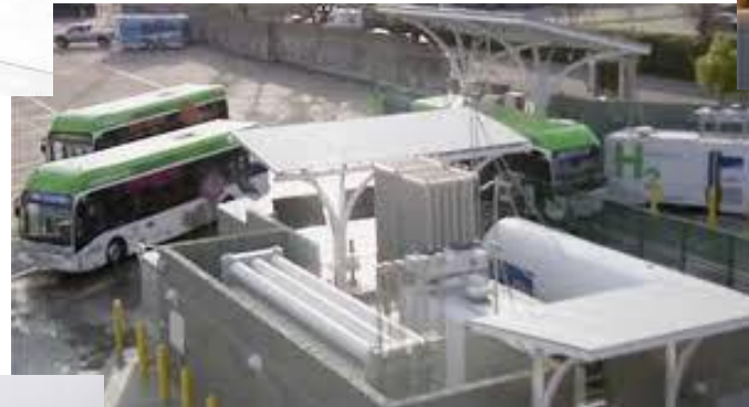
AC Rapid Transit Oakland, CA Site Generated & Delivered H2
