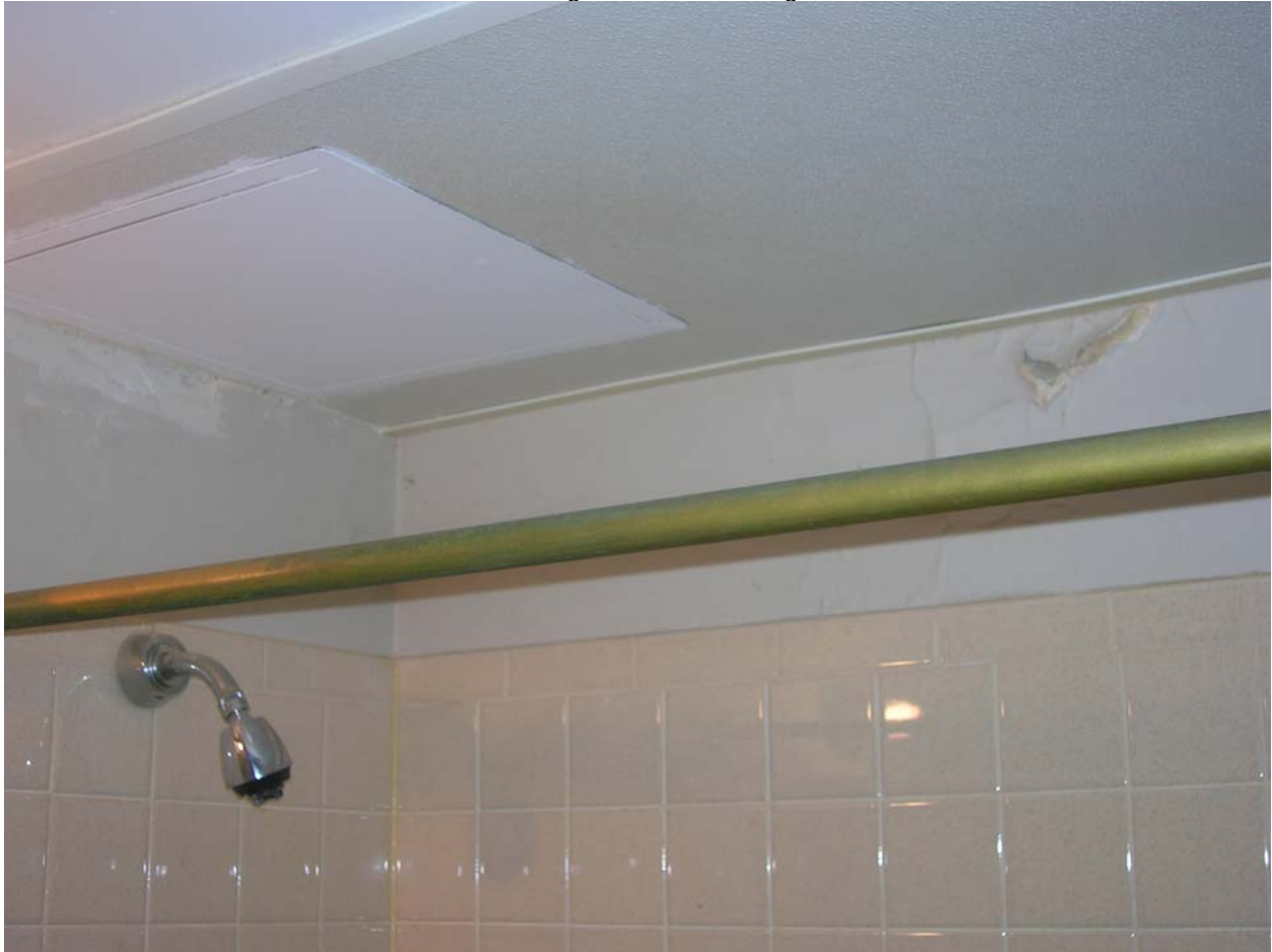
200-1 Family Housing Development 13 Tudor Street Cracked and Damaged Bathroom Ceiling and Walls
