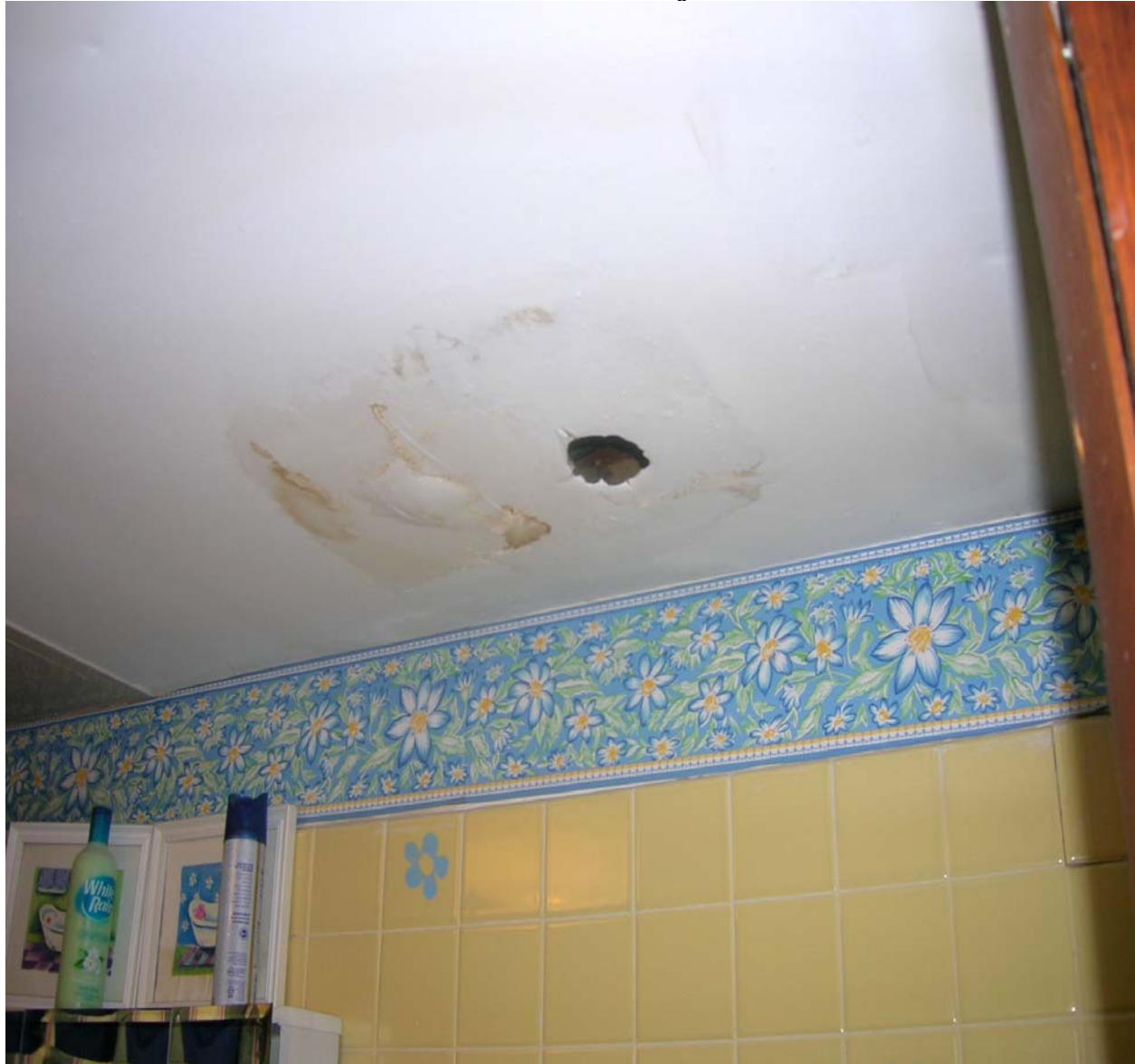
689-1 Development 26 Haverhill Street Hole in Bathroom Ceiling
