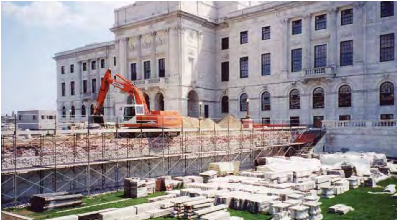
Project: Rhode Island State House Location: Providence, RI Completion Date: 2010 Client: State of Rhode Island Client Contact: Arthur Jochmann 401.222.1285
