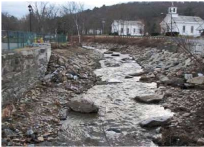
Boulders placed along the edge of restored stream channel to enhance fish passage upon removal of Ballou Dam in Becket, MA
