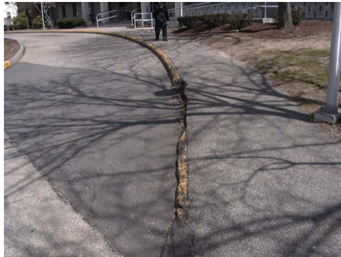
667-2 Woodland Towers – Sidewalks Need Repair or Replacement
