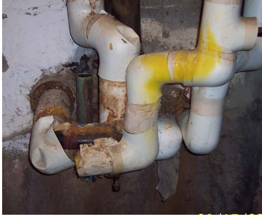
200-1 Lexington Gardens – Water Pipes are Rusting and Leaking Water
