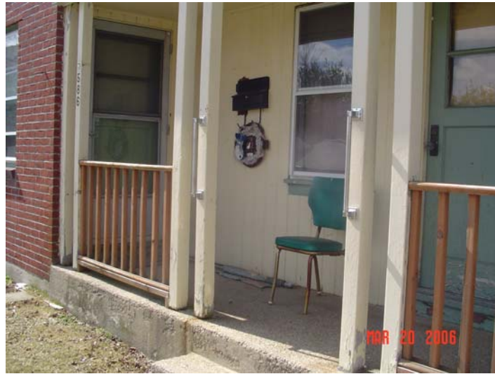
667-1 Elderly Housing Development, Crestview Building Exterior – Peeling and Rotting Porch Posts
