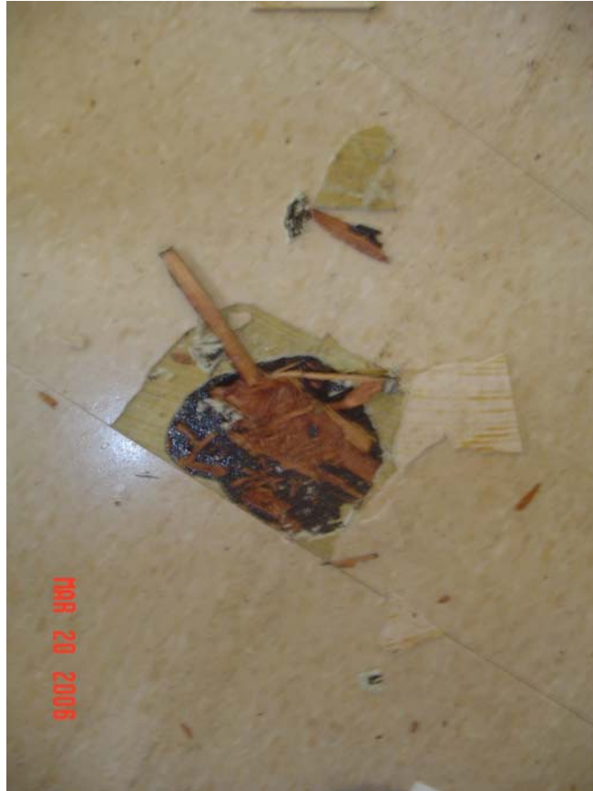
667-1 Elderly Housing Development, Crestview, 592 Summer Street Bathroom – Cracking and Lifting Floor Tiles
