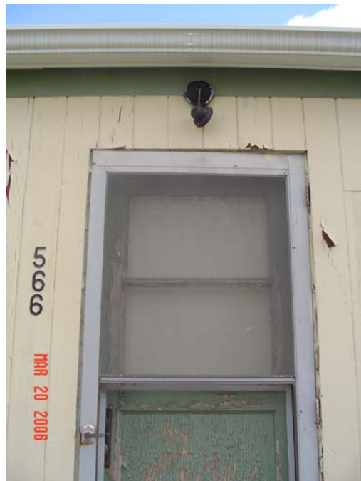
667-1 Elderly Housing Development, Crestview, 592 Summer Street Building Exterior – Main Door Peeling and Rotting, Screen Door Frame Rotting, and Screen Window Missing
