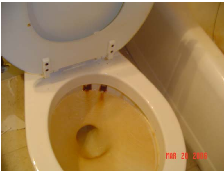
667-1 Elderly Housing Development, Crestview, 592 Summer Street Bathroom – Rusty Water
