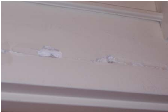
667-2 Development, Edwin Seibel Apartments Common Area – Plaster Crumbling Around Doorframe
