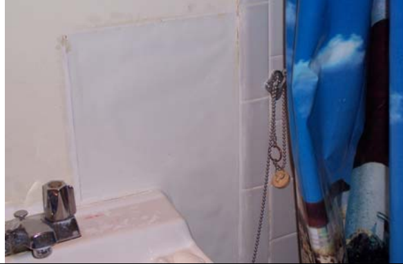
667-2 Development, Edwin Seibel Apartments Bathroom – Wall Behind Tile Is Deteriorating
