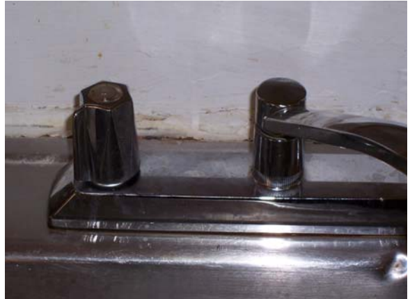
705 Development, Scattered Sites Dented Sink and Water Damage on Wall Behind Faucet in Kitchen
