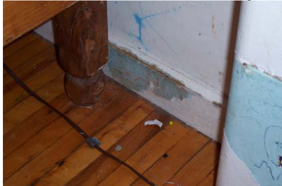
200-1 Development, Beaudoin Village Bedroom – Baseboard Paint Peeling
