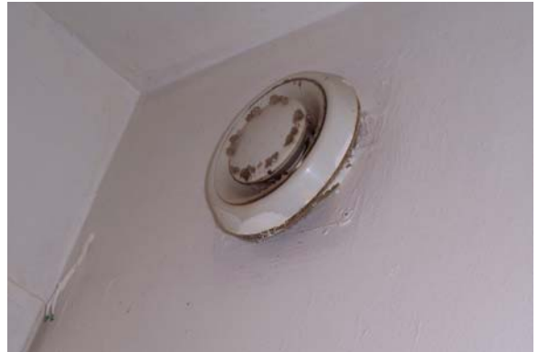
705 Development, Scattered Sites Bathroom - Mold and Mildew on Exhaust Fan
