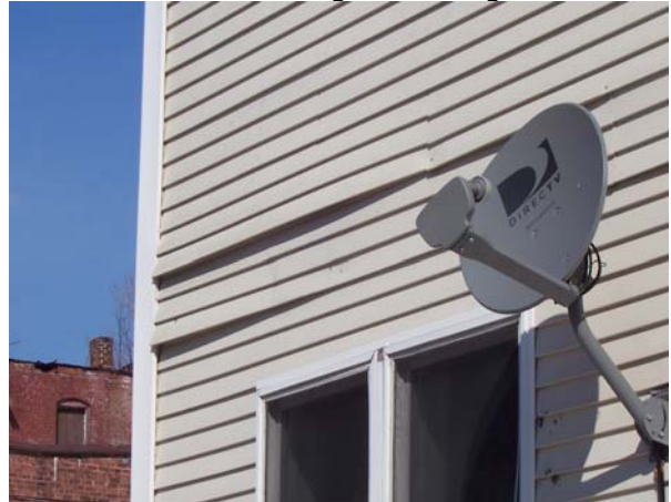
705 Development, Scattered Sites Loose Siding on Building
