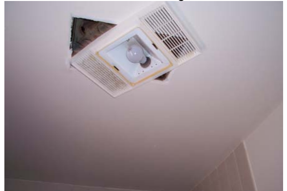
705 Development, Scattered Sites Bathroom – Vent Cover Hanging and Light Fixture Cover Missing
