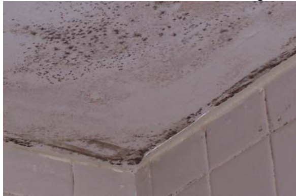
705 Development, Scattered Sites Mold and Mildew on Bathroom Ceiling
