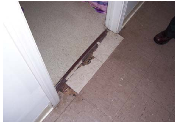
705 Development, Scattered Sites Cracks, Tears, and Missing Pieces in Floors in Common Area
