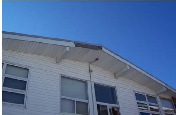
667-2 Development, Edwin Seibel Apartments Piece of Fascia Missing
