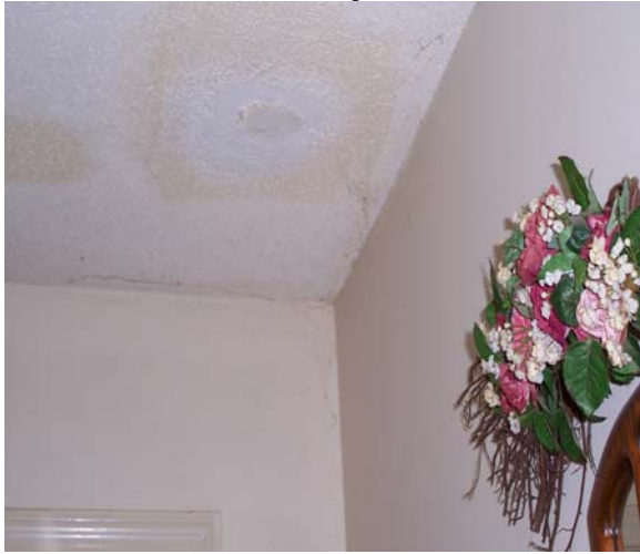
705 Development, Scattered Sites Common Area – Patched Ceiling due to Water Damage
