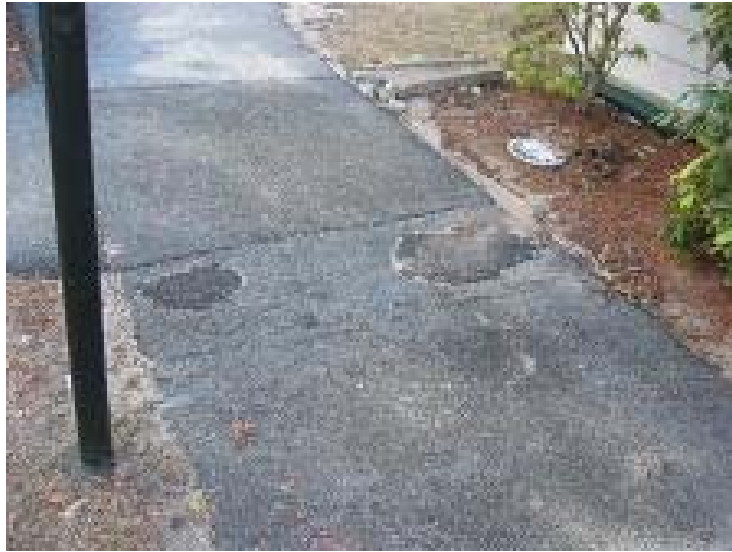
667-1 Elderly Housing Development, 14E Birchcrest Street Outside Area – Sinkholes Forming on Sidewalks
