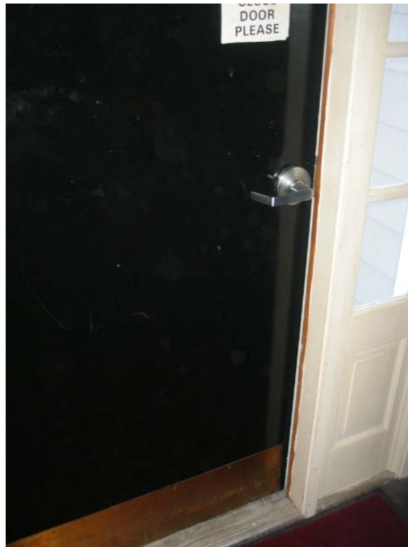
667-1 Elderly Housing Development, 14E Birchcrest Street Entrance – Security Door Does Not Close Properly
