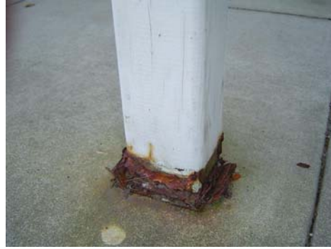
Project 667-1 Rusted and Rotted Support Post
