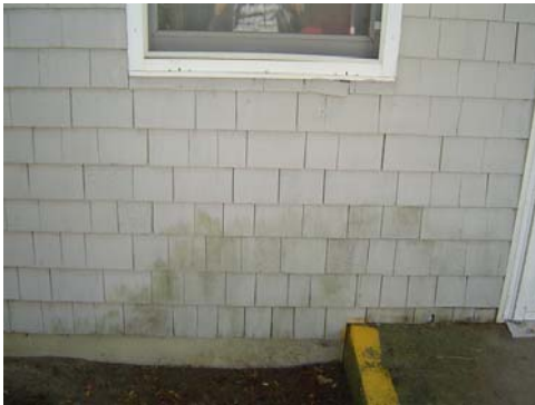
Project 667-1 Mold and Mildew on Exterior Shingles
