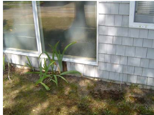
Project 667-1 Missing Exterior Shingles
