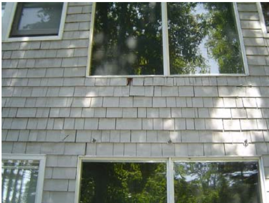
Project 667-1 Missing Exterior Shingles
