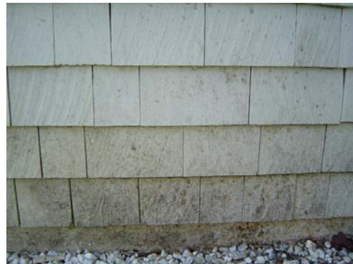
Project 667-1 Mold and Mildew on Exterior Shingles
