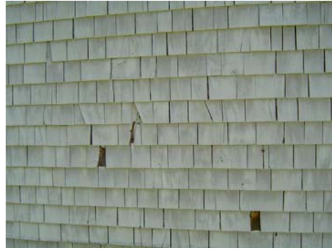
Project 705-1 Broken and Missing Shingles
