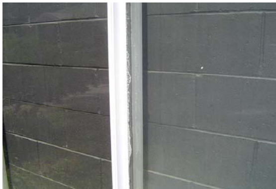
Project 667-1 Shattered Glass Slider with Concrete Block Wall
