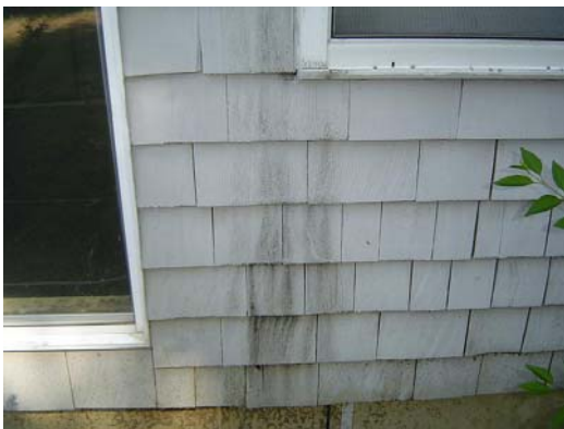
Project 667-1 Mold, Mildew on Exterior Shingles
