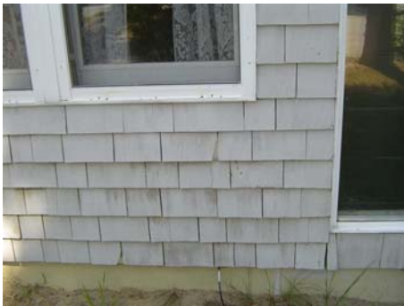
Project 667-1 Broken Shingles
