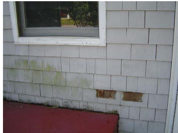
Project 667-1 Mold, Mildew, and Missing Paint on Exterior Shingles
