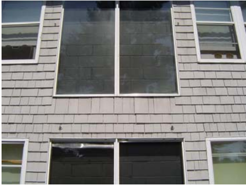
Project 667-1 Missing Row of Exterior Shingles
