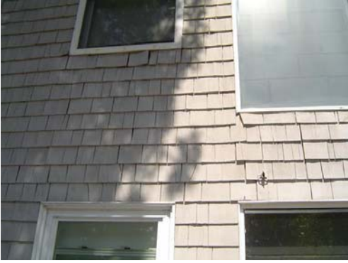
Project 667-1 Broken Exterior Shingles
