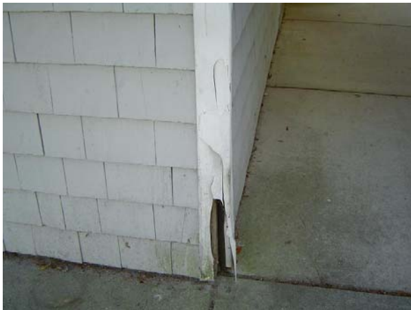
Project 667-1 Rotted Corner Post
