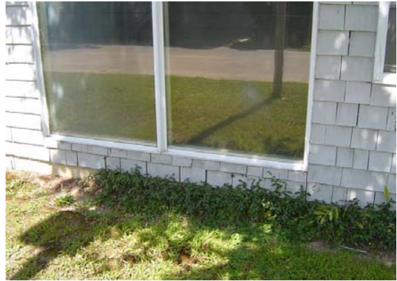
Project 667-1 Missing Exterior Shingles
