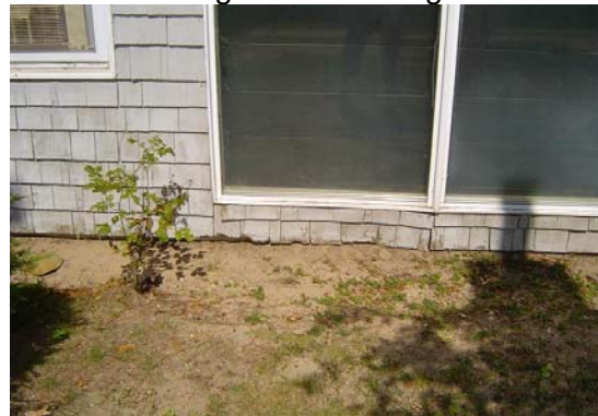
Project 667-1 Rotted Exterior Shingles
