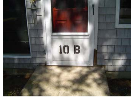
Project 667-1 Rotted Exterior Door Casing
