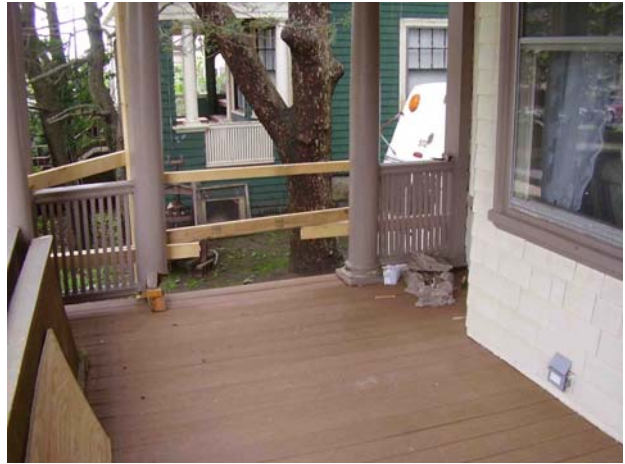
386 Broadway - Missing front porch railings, makeshift railing
