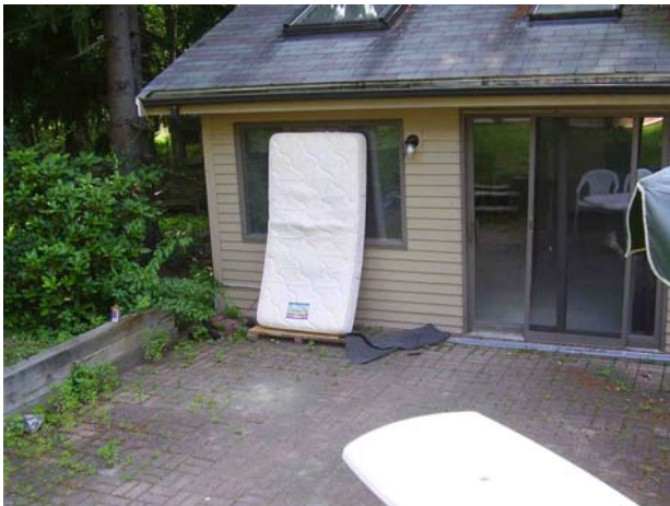
Overgrown foliage, roof and screens in need of repair
