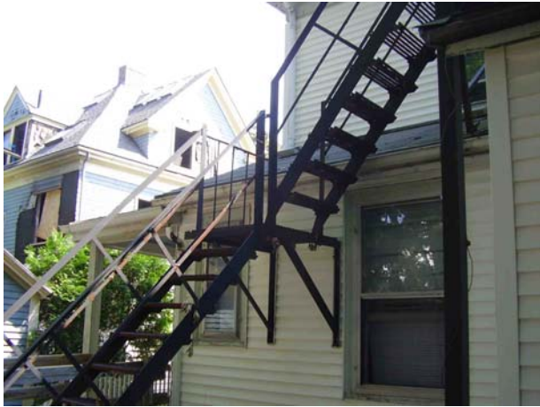
Old and rusty fire escape
