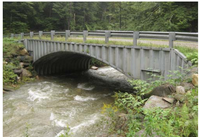
The upstream end of a bottomless culvert on Bronson Brook, that DER helped install, post-Tropical Storm Irene. Crossings of this type faired well in the high flows.
