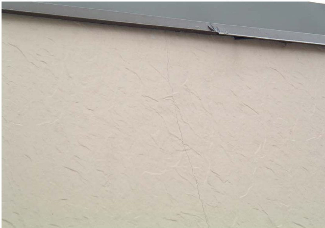
667-3 Elderly Housing Development, 506 Pope Towers Building – Separated Flashing
