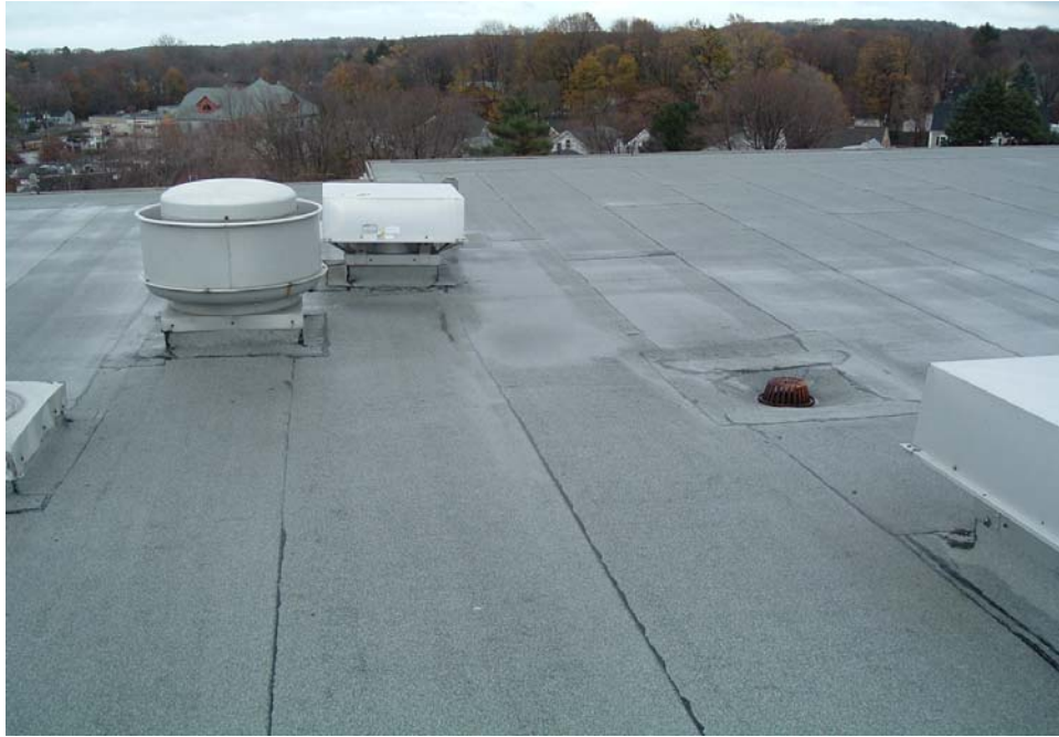
667-3 Elderly Housing Development, 506 Pope Towers Building –Roof Vents Do Not Remove Moisture
