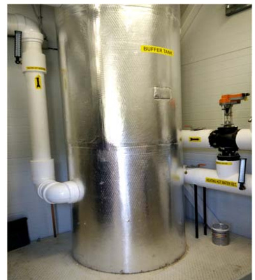
Thermal storage tank
