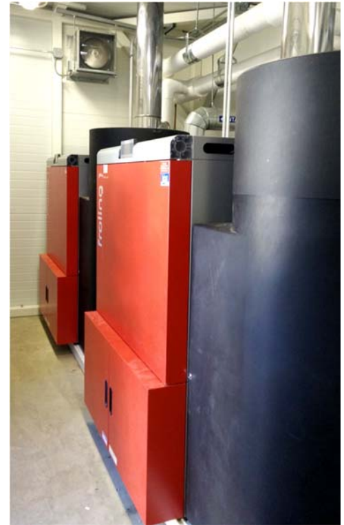
Wood pellet boilers
