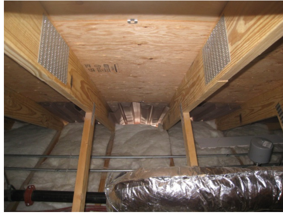
Figure 10 - Wind baffles installed without proper sealing, not code compliant
