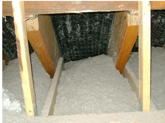
Figure 5 - Blown cellulose attic insulation
