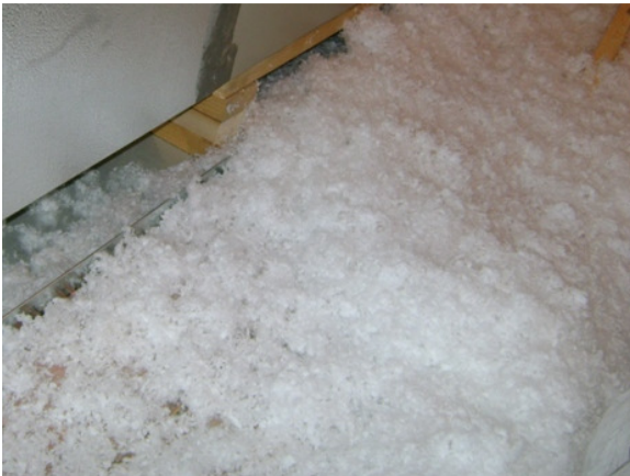
Figure 4 - Blown fiberglass attic insulation
