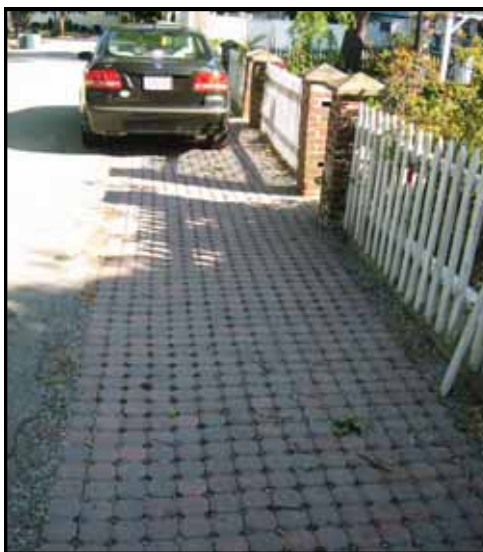
Permeable pavers along Silver Lake Ave. sit on top of stone beds that capture and filter runoff and allow it to soak into the ground.
