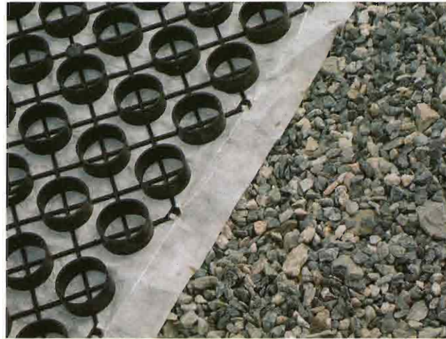
One of two porous paving systems installed in an overflow parking lot, GravelPave consists of gravel contained in small plastic containers that provide structural integrity.
