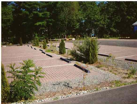
Permeable interlocking concrete pavement units, also known as porous pavers, were installed within the parking spaces at the Silver Lake town beach, and multiple bioretention cells were constructed along the perimeter and as a central traffic island.
