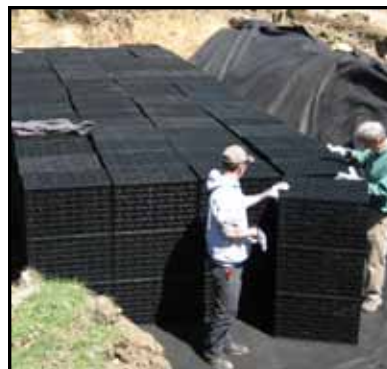
8000-gallon vault system at the Boutwell School that captures rainwater for irrigating athletic fields.
