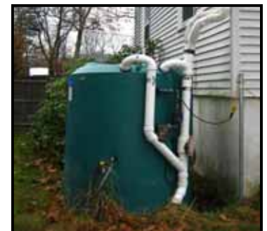
200-gallon (top) and 800-gallon (bottom) rainwater harvesting systems were installed at 39 residences.
