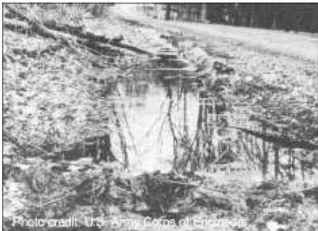
Obstructions in this ditch have led to standing water
