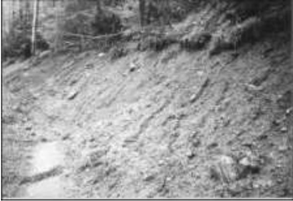
1. Before the project, the roadside bank was severely eroding which led to continual maintenance.
