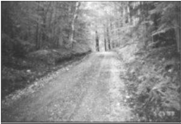
1. Before the project, Tyringham Road was narrow with steep banks and no formal ditches.
