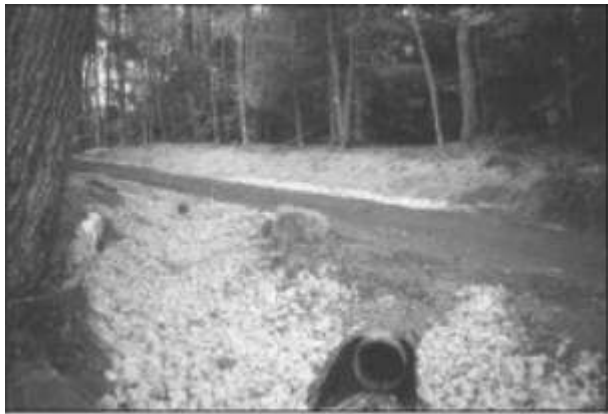
3. To improve the drainage, ditches were constructed on both sides of the road and culverts were used to direct water to stable outlets.
