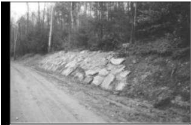
3. A Work in Progress: To stabilize the bank, the town used a combination of small and large rocks on the face of the bank. A ditch was constructed along the toe of the slope and culverts were used to direct runoff to stable outlets before it reached the river.
