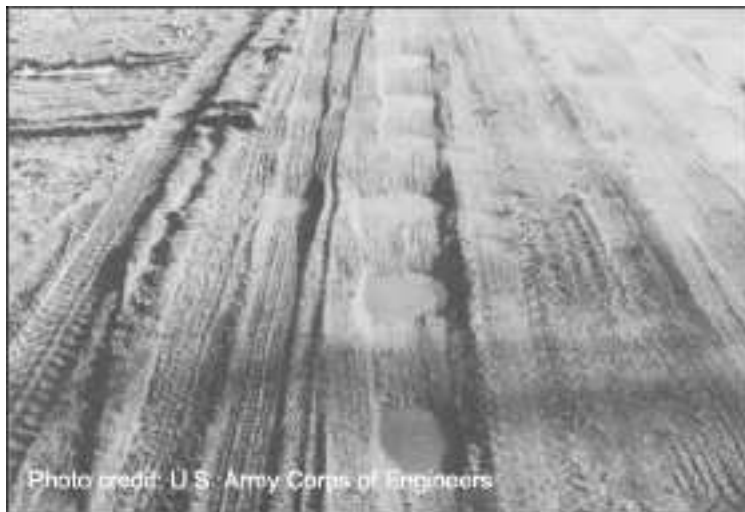
Corrugations on an unpaved roadway
