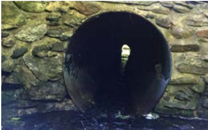
Brookfield received a DER grant to replace this undersized culvert.
