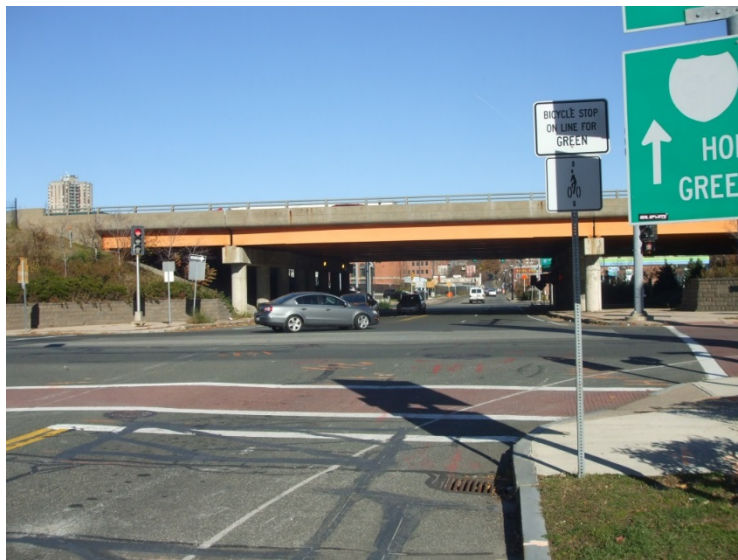
Figure 2-43: West Columbus Avenue (Hall of Fame Avenue) at Union Street – Pavement marking symbols and interstate shield at the eastbound approach are worn.
