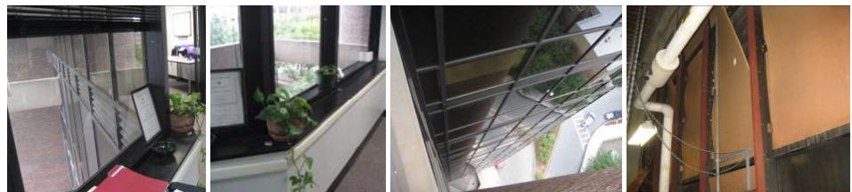
L&CL (Left & Center Left Photos)- Many of the exterior louvers are ornamental. CR (Center Right Photo)- uninsulated curtain wall with single pane glass. R- Mechanical room glasses are painted and insulating board added but is falling apart.
