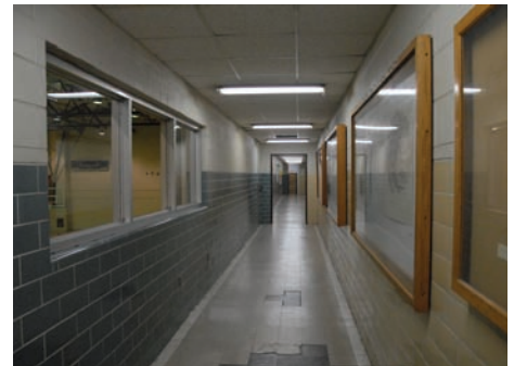
The Gymnasium, with its huge, largely unused volume of space and ineffective internal circulation, is a fitting site for redevelopment
