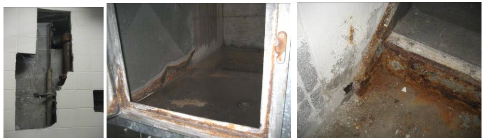
L- Showing opened up wall cavity necessitated to repair numerous freeze-up problems. C- Lobby unit AHU is located in basement; this shows an outside intake plenum connected to an areaway... street water comes in overloads the drain and readily pours into the mechanical room. R- Shows severe corroded state of basement stairs just outside the mechanical room, an evidence of years of flooding problem virtually during every heavy rain.
