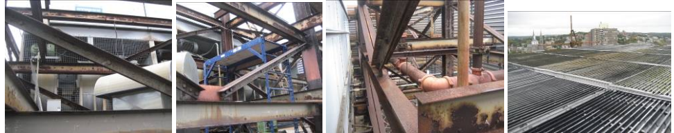
L&CL- 3 cell Evapco LSTA10-364 (s/n 952303; 3 x 60-HP fan motors) nominal 1,000-ton capacity (needs to be confirmed) forced draft cooling tower was installed 10 years ago within the existing structure to replace the old tower. One fan motor was just replaced. Condenser water piping is the original and are showing numerous leakages.
