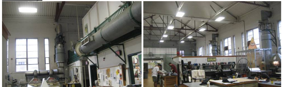
Entire upper level is the Print Making Room. L- Note the heated and ventilated supply ductwork along the right wall; note the source capture exhaust hoods over printing devices
