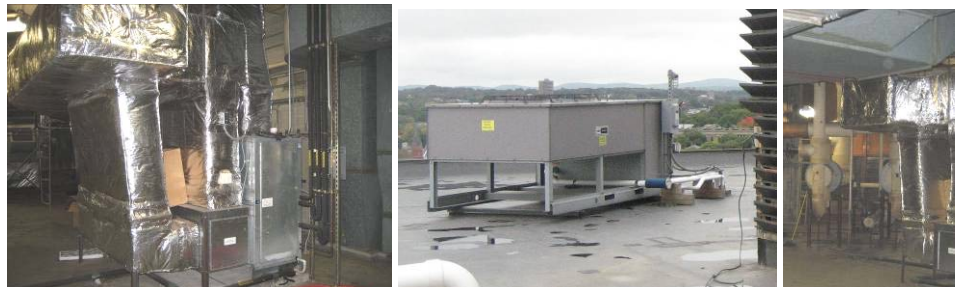
L&CL- new elevator machine room 25-ton Carrier split DX AC system. CR- two steam to hot water converters; one for perimeter and one for reheat.
