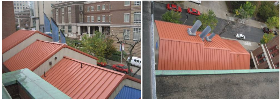
Roof view of the Glass Hot Shop. Note the 3 exhaust fan stacks. This project was one of the earlier DCAM design-build project, using pre-engineered metal building. Mechanical Engineer of record was VAV Int'l.
