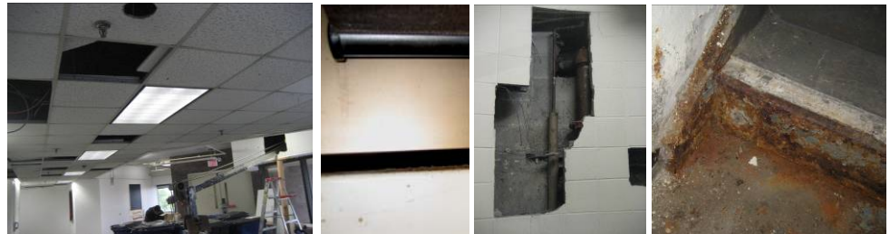
L- Many parts of building have ceiling tiles in very poor shape. CL- unit ventilators are not sealed against its louvers... most often there's 1/2" gap with huge rate of outside air infiltration. CR- one of many evidence of frozen pipes in wall spaces caused by negative pressure induced cold air infiltration. R- Basement bottom stairs is badly corroded from water flooding in through areaway air intake virtually every time it rains.
