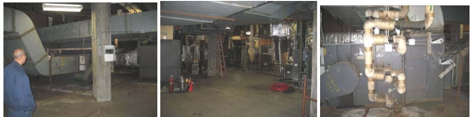
L, C & R- Penthouse MER showing the 30 year old constant volume air handling units AC-11 and AC-12 in poor shape. AC-11 serves the South Pod from 8 th through 13 th floors while AC-12 serves the North Pod on floors 8 through 10. These interior parts of the building are served by antiquated and energy wasting constant volume reheat system.
