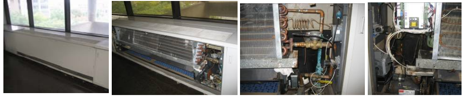
L- Typical 4-pipe unit ventilator (UV). CL- UV with front panel removed showed that it is in a remarkable shape, testament to extraordinary maintenance. CR- 2W pneumatic ACV with E-P transducer to interface to DDC system, Belimo electric actuator for dampers, and bus to DDC network; note that valves and pipes are uninsulated and does not have auxiliary pan to catch the condensate drips. R- Automated Logic DDC board.
