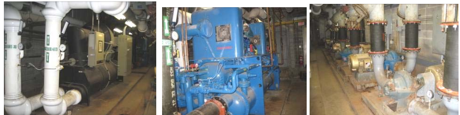
L- Trane 420-ton electric centrifugal chiller. C- TecoChill gas fired engine driven chiller; it is a twin set of two GM V8 based automotive engine each driving a screw compressor; had very troublesome record for first few years but now is fixed and operational but requires very high maintenance. Both chillers were installed 10 years ago to replace the original two 500-ton steam absorption chillers; only one needs to run on a partial load to meet Tower Building and North Building Auditorium cooling demands. R- 6 pumps; 3 chilled water pumps each at 50-HP; 3 condenser water pumps each at 60-HP.
