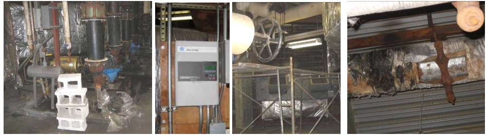
L- 3 hot water pumps; one for perimeter unit ventilators, one for reheat, and one for spare. CL- an A-B VFD for one of the HW pump. CR- one of two ventilation fan. R- Showing piping insulation in a very poor condition and showing condensation drips.
