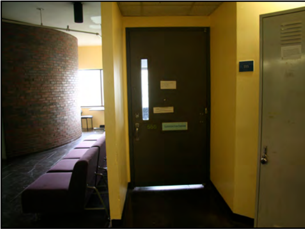
LOCATION | 514 (T555 no latch pull side clearance)
