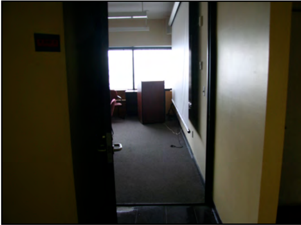
LOCATION | 516 (T555 no latch pull side clearance)
