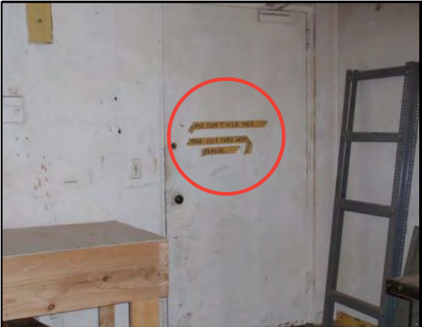
FIG. EAST - Basement egress signage hand-written on masking tape that is peeling off
