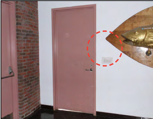
FIG.2 TOWER - 8th Floor missing signage
