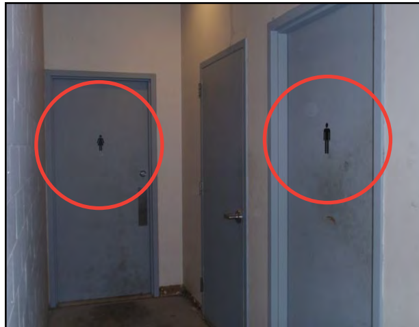
FIG. EAST - 1st Floor non-compliant toilet
