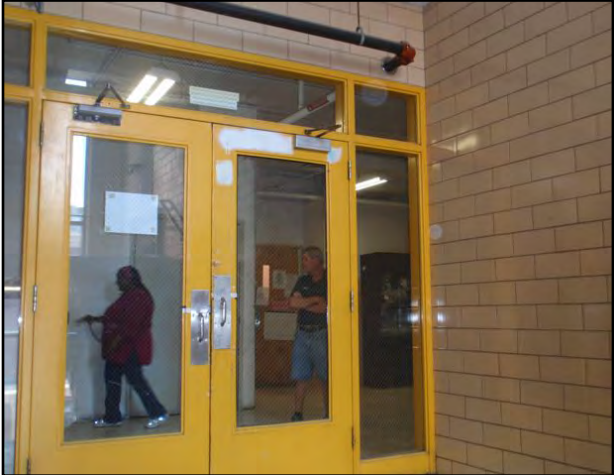
FIG.1 KENNEDY - 3rd Floor signage missing
