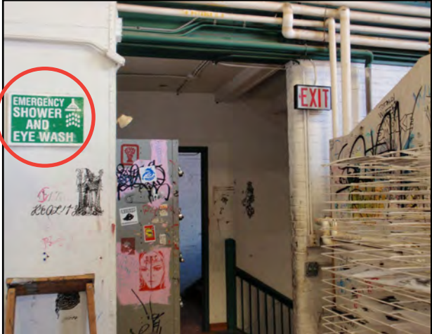
FIG.8 EAST - 2nd Floor - signage ADA non-compliant
