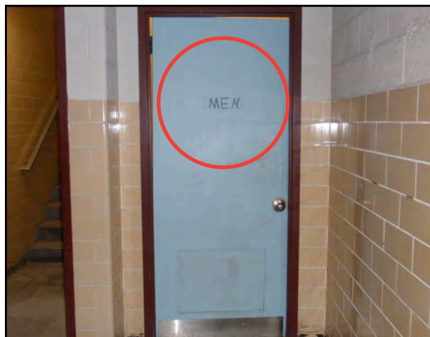
FIG. EAST - Basement handwritten non-compliant toilet room signage
