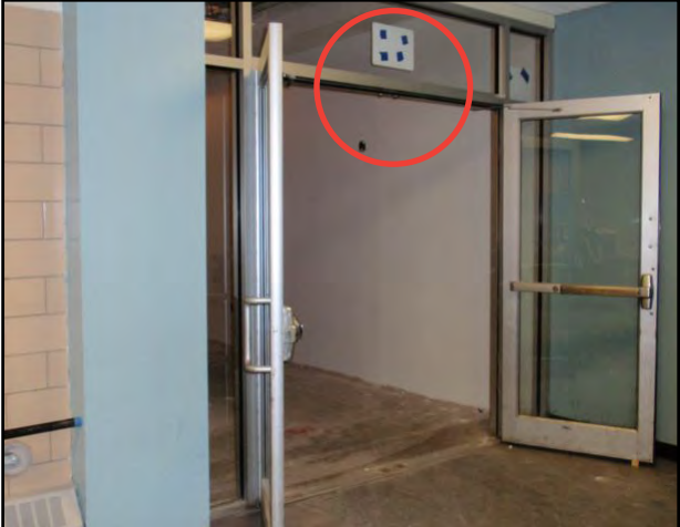
FIG.9 SOUTH - 2nd Floor - Signage missing
