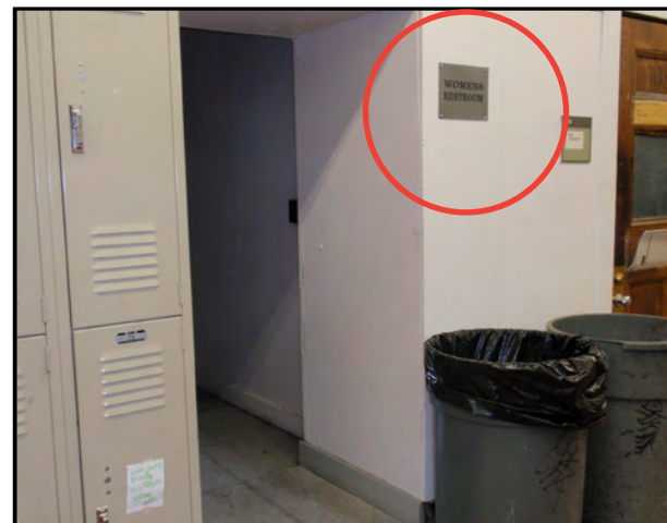
FIG.SOUTH 2nd Floor non-compliant toilet
