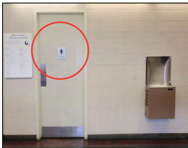
FIG.TOWER - 12th Floor non-compliant toi-
