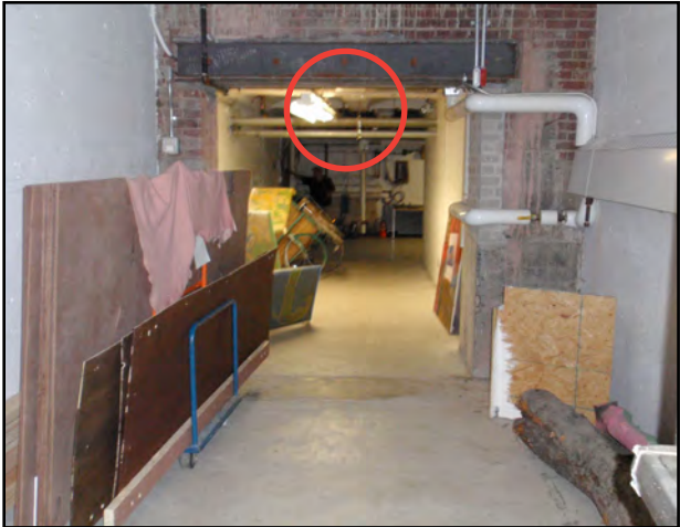
FIG. NORTH - Basement Exit sign cannot be seen as it is obstructed by plumbing
