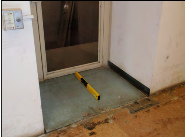
LOCATION | B10/208 Lift
