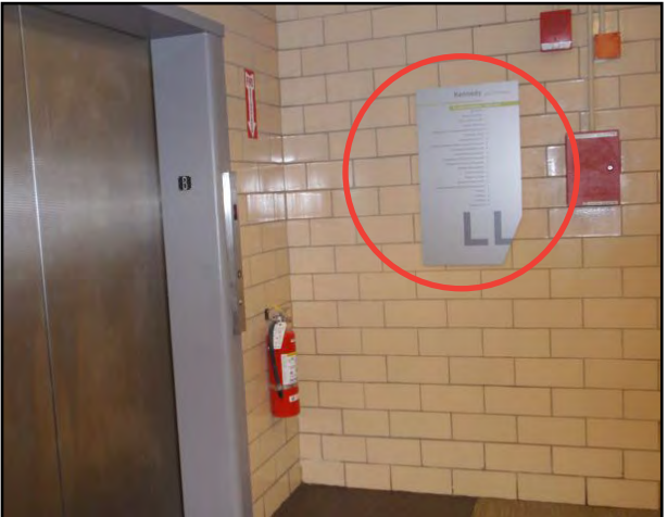
FIG.6 KENNEDY - Basement Elevator Lobby Directory confusing & non-compliant for text height and contrast
