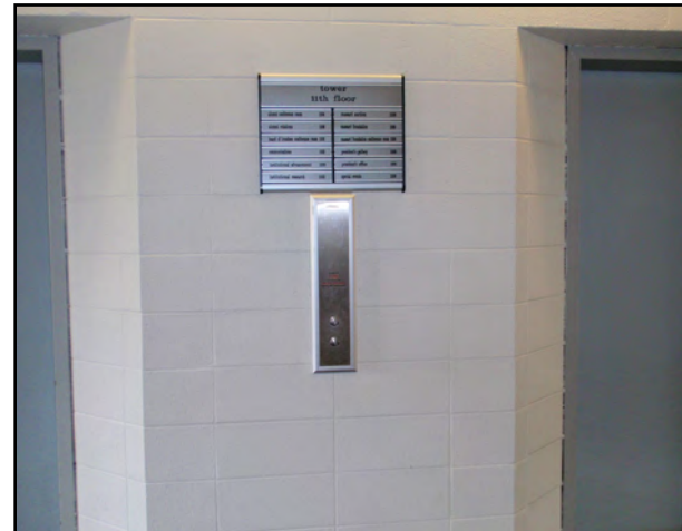
FIG. TOWER- 11th Floor Elevator Lobby Directory is too high. Height makes it difficult for a seated person to read
