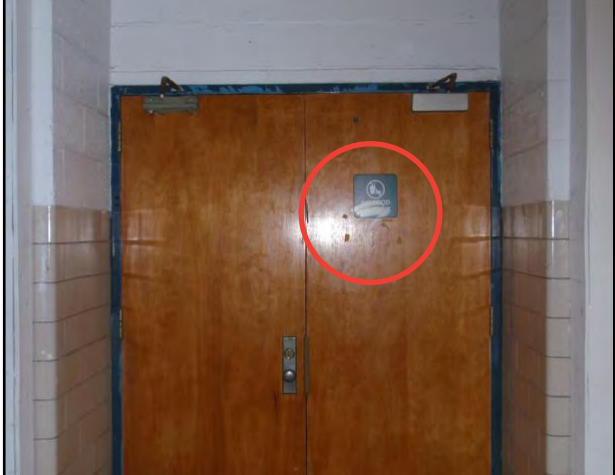
FIG.2 KENNEDY - 4th Floor signage ADA non-compliant
