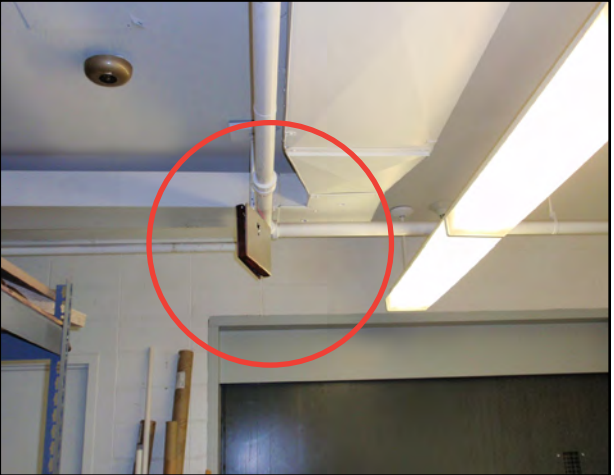
FIG. TOWER - 10th Floor exit sign as been turned to face wall so it can't be seen.
