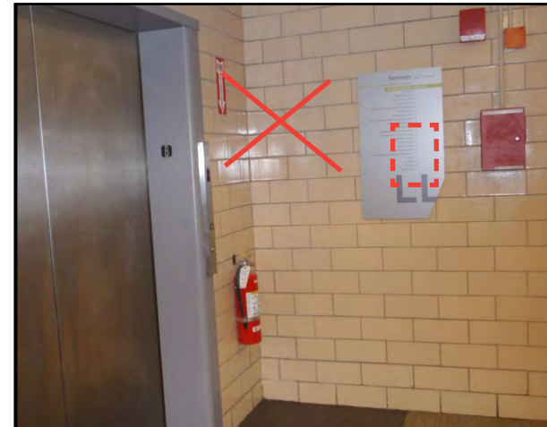
FIG. KENNEDY - Basement elevator lobby new directory confusing, non-compliant for text height, contrast & content not coord.
