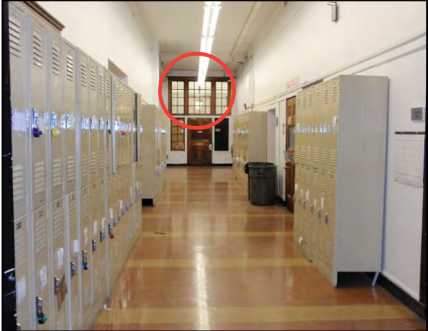
FIG. SOUTH - 2nd Floor exit sign missing
