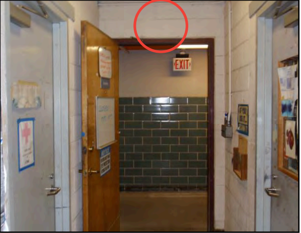
FIG. EAST - Basement exit sign missing in room
