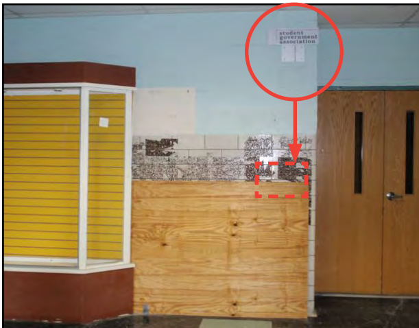
FIG.8 KENNEDY - 2nd Floor signage too high and non-compliant for character pro-
