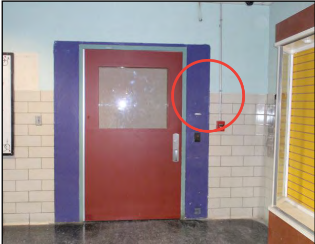
FIG.7 KENNEDY - 2nd Floor signage missing
