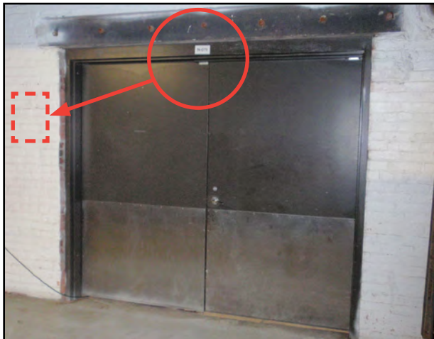
FIG.4 NORTH BASEMENT - Storage signage wrong location and non-compliant for character proportion and size
