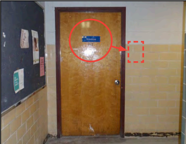
FIG.3 EAST - Basement Woodshop wrong location and non-compliant for character proportion and size
