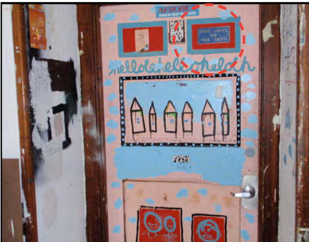
FIG.9 NORTH - 2nd Floor "doors locked for your safety" signage too high and non-compliant for character proportion and size
