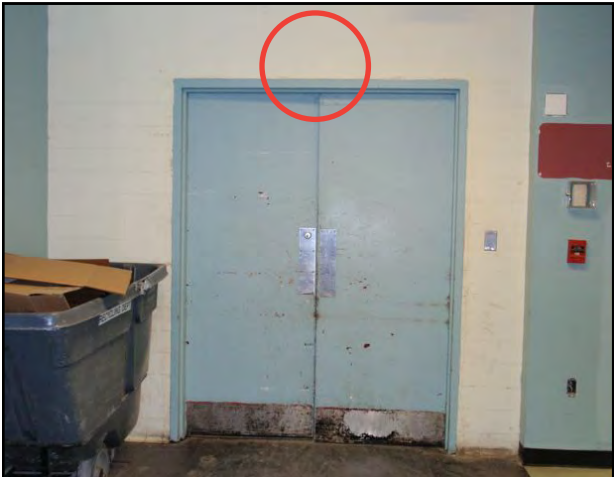
FIG. SOUTH - 2nd Floor exit sign missing
