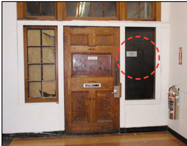
FIG.5 SOUTH - 2nd Floor wrong location and non-compliant for character proportion and size
