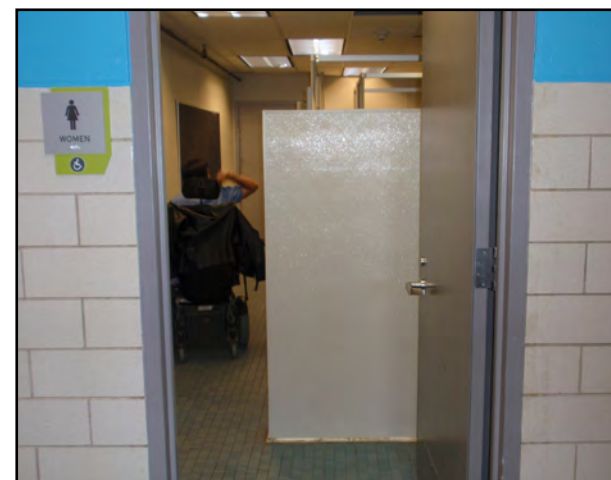
FIG KENNEDY - Basement non-compliant
