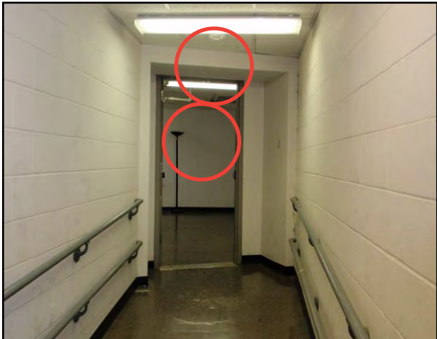
FIG. BETWEEN TOWER & EAST - 2nd Floor exit sign missing
