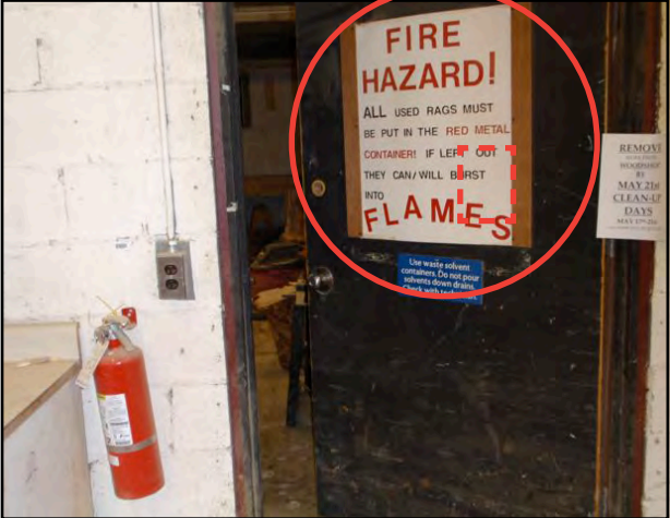
FIG.3 EAST - Basement Woodshop-signage ADA non-compliant
