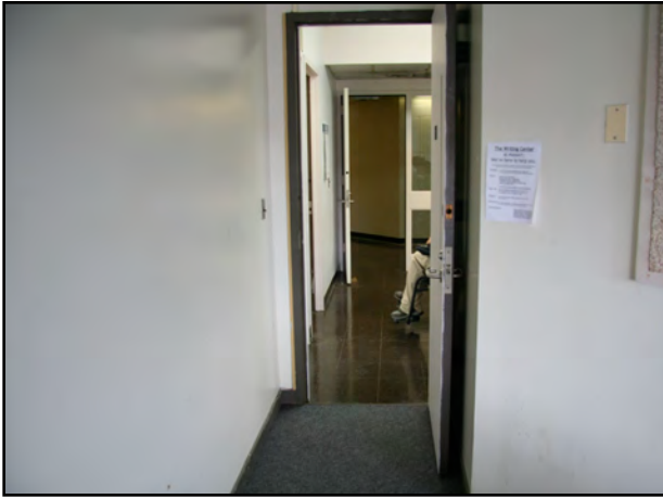
LOCATION | 503 (T552 no latch pull side clearance)
