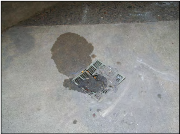
LOCATION | X26 Bottom of Tower Ramp - hazard to ramp users
