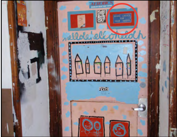
FIG. NORTH - 2nd Floor "doors locked for your safety" signage too high and non-compliant for character proportion and size
