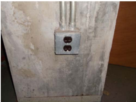
Figure 2.8.4: Receptacles are original and beyond their useful service life.
