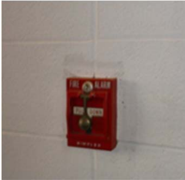
Figure 2.8.10 Existing fire alarm devices
