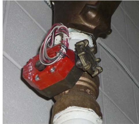
Figure 3.3.6 Fire alarm device not connected to fire alarm system
