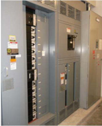
Figure 2.8.6 Several pieces of emergency electrical distribution equipment were replaced around 1999 and are in good condition.
