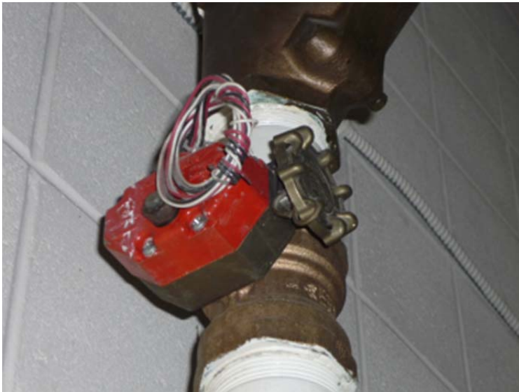
Figure 2.10.6. Flow switch not connected to fire alarm.
