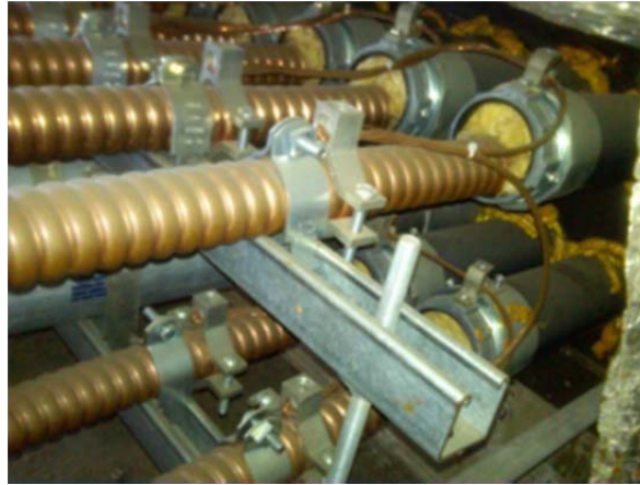
Figure 2.8.7 MI cable installed for emergency loads.
