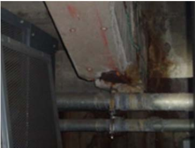
Figure 2.4.26 Beam in Electrical Transformer Room
