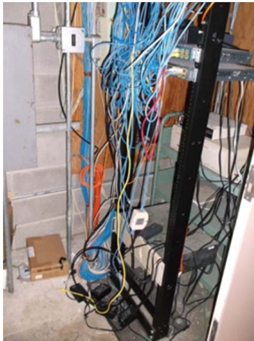
Figure 2.8.16 Typical telecomm closet with a mixture of newer and older patch panels and cabling
