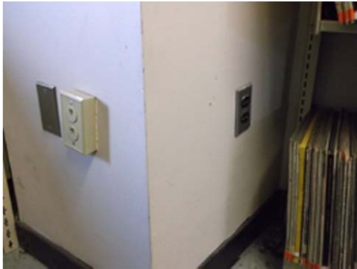
Figure 2.8.14 Existing telephone outlets are original and beyond their service life.
