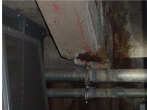
Figure 3.3.11 Fire pump corroded casing and supports
