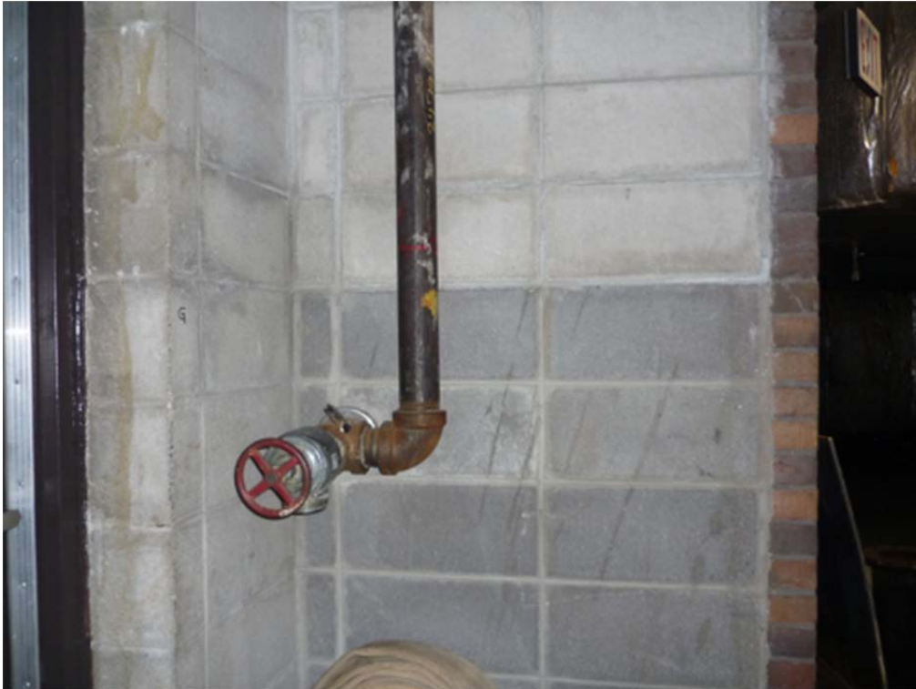
Figure 2.10.4. Hose valve connection at Level 14
