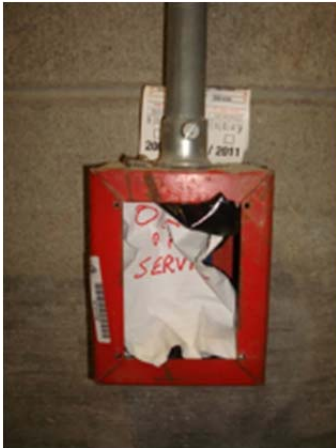
Figure 2.8.12 Existing fire alarm device appears to be abandoned.
