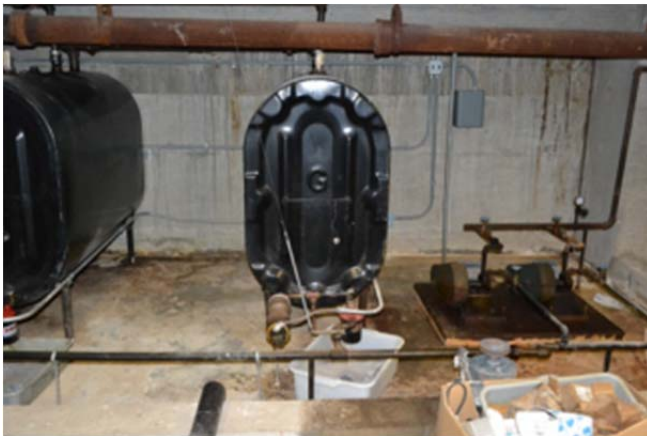
Figure 2.7.5 Diesel storage tanks
