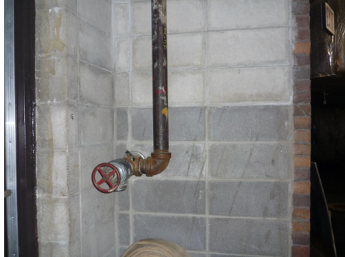
Figure 3.3.5 Hose valve connection outside the stair enclosure
