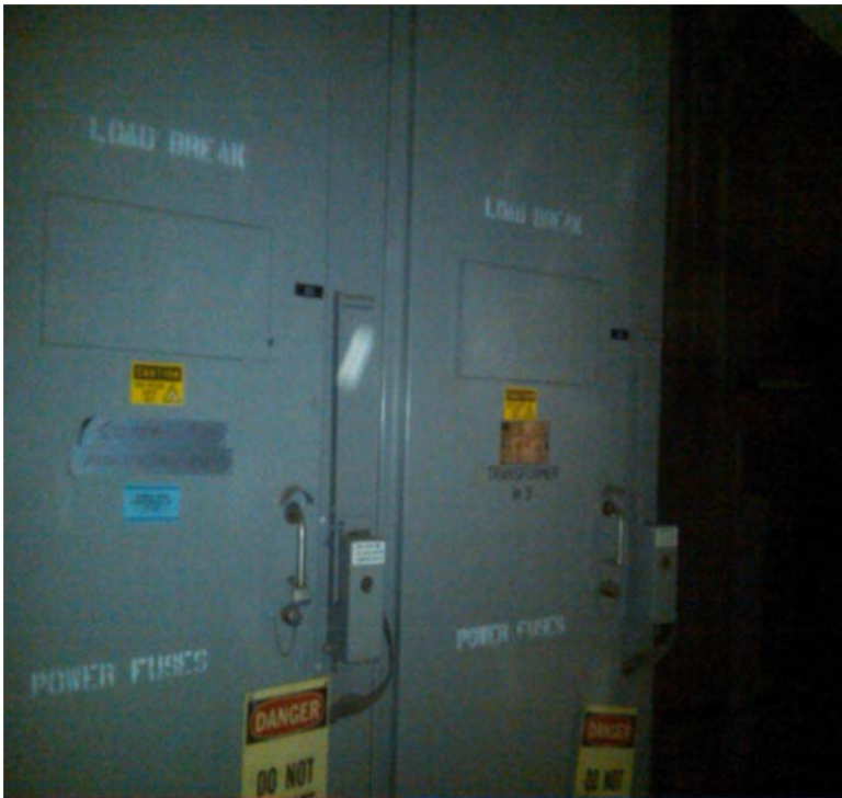
Figure 2.8.1: Existing utility owned 15kV switchgear
