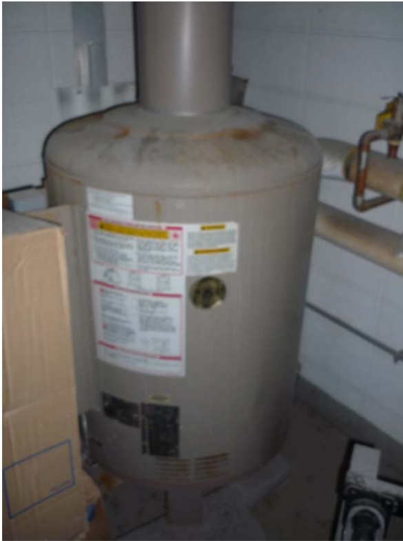
Figure 2.9.3 Gas fired water heater
