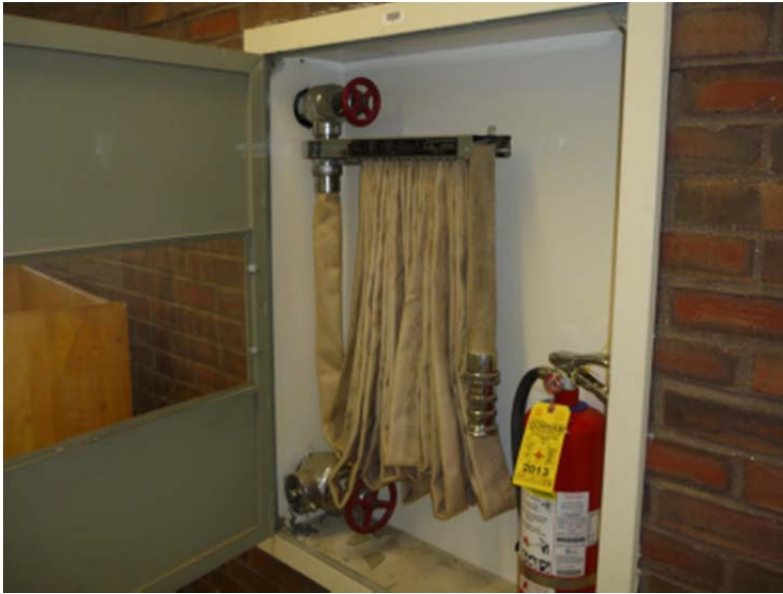
Figure 2.10.5. Hose valve cabinet with hose reel
