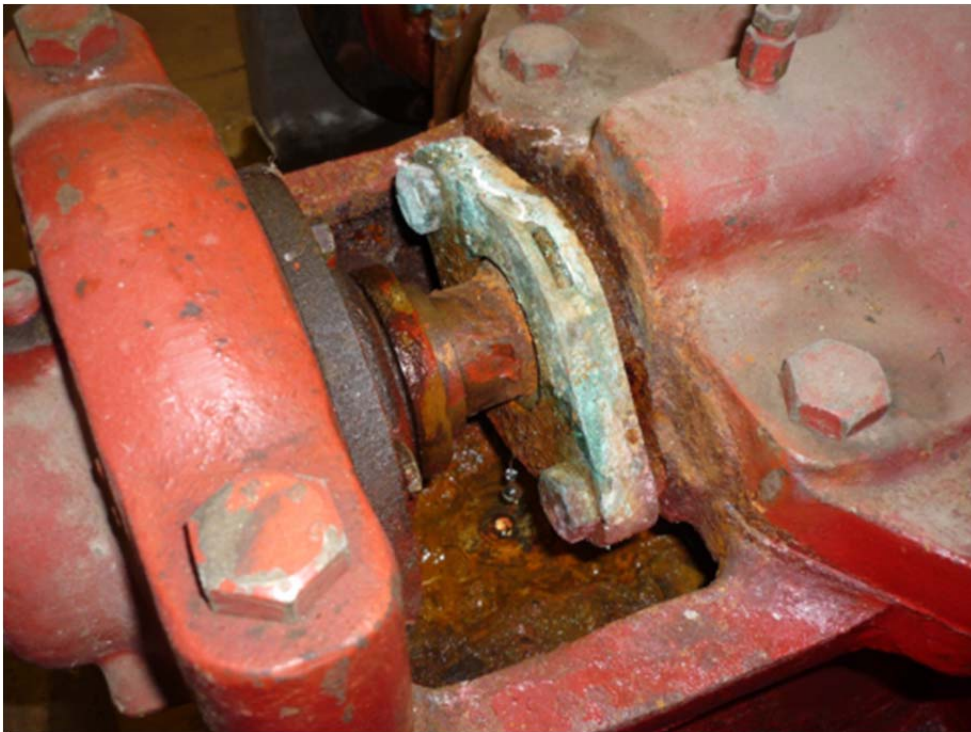
Figure 2.10.2 Fire pump leaking from casing
