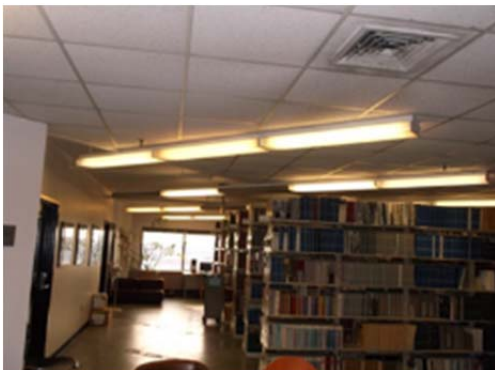
Figure 2.8.8 Existing light fixtures are original and are beyond their useful service life
