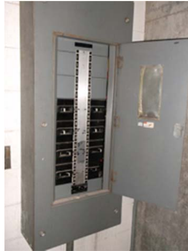
Figure 2.8.3 Typical FPE panelboard is old and beyond its useful service life.
