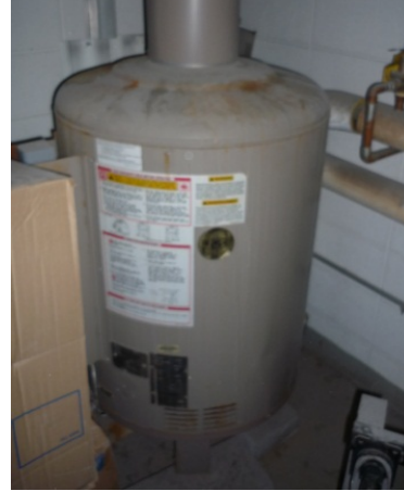
Figure 3.3.8 Gas fired water heater with 180°F leaving water
