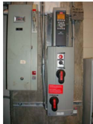
Figure 2.8.5: Some newer VFD's and motor controllers have been installed over the years.
