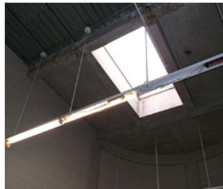
Figure 2.8.9 Some light fixtures are missing lenses and falling apart.
