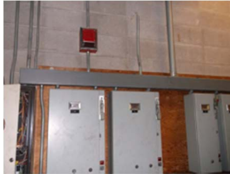
Figure 2.8.11 Fire alarm wiring is routed in raceway used for power wiring.
