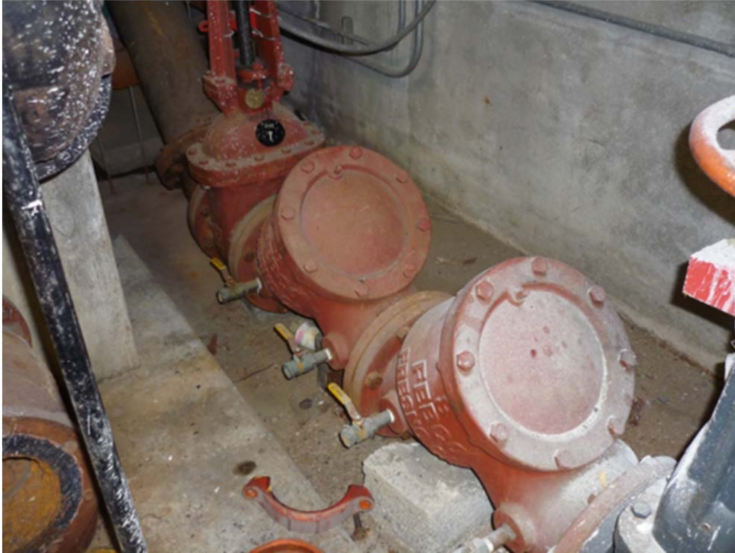
Figure 2.10.1 Incoming 8" fire main with double backflow preventer.
