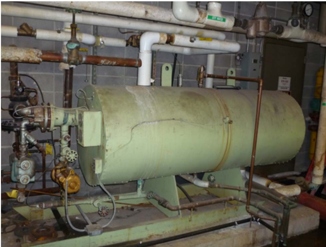
Figure 2.9.2 Original steam water heater
