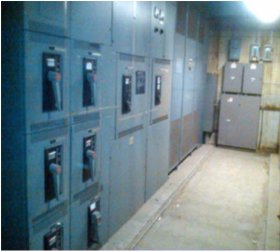
Figure 2.8.2: Existing MCAD Switchboard is old and beyond its useful service life.
