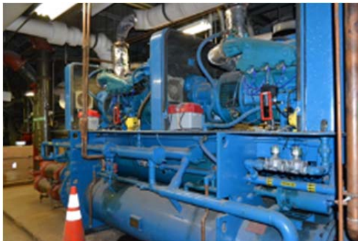
Figure 2.7.2 Chiller plant, Thermo Corp chiller shown
