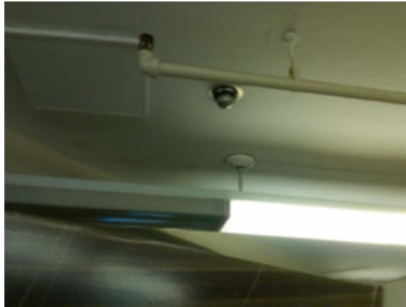
Figure 2.8.13 Existing original heat detectors are still being used and are beyond their useful service life.
