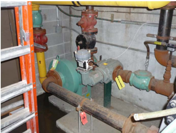
Figure 2.9.4 Incoming gas main and booster.
