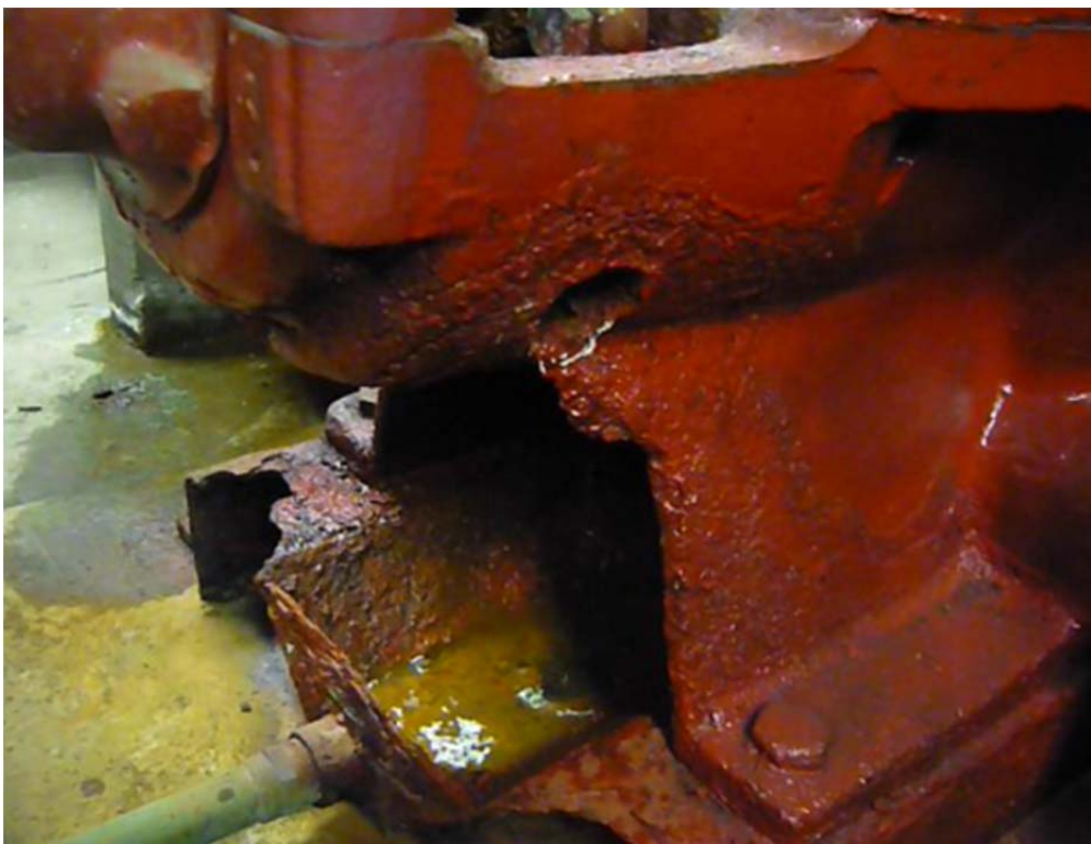
Figure 2.10.3 Corroded casing and supports for the fire pump
