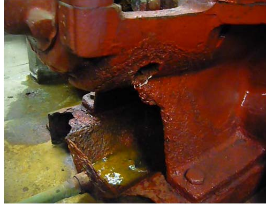
Figure 3.3.7 Fire pump corroded casing and supports
