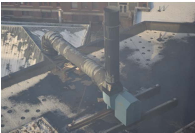
Figure 2.7.8 Wood shop exhaust
