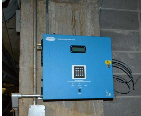
Figure 3.3.9 Existing Refrigerant Monitor Panel
