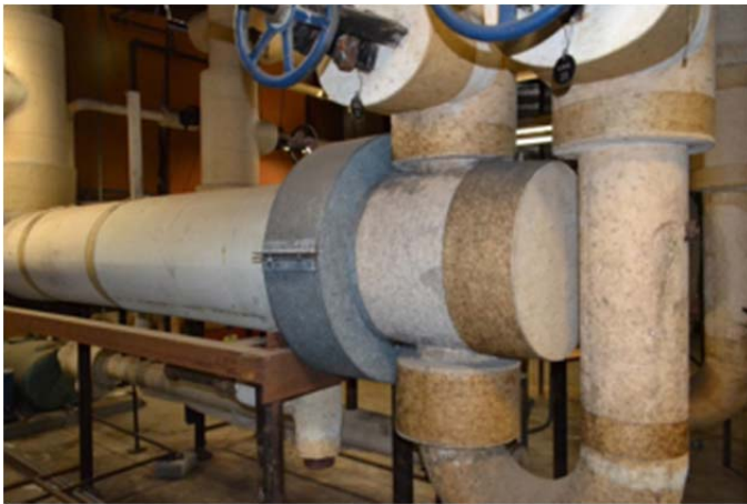
Figure 2.7.1 Steam to HHW heat exchangers
