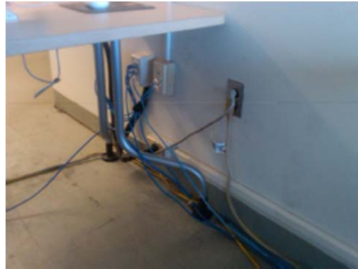
Figure 2.8.15 Surface mounted tel/data outlets and surface raceway have been installed over the years.
