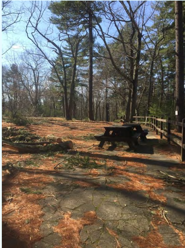
Existing pavements in poor condition
