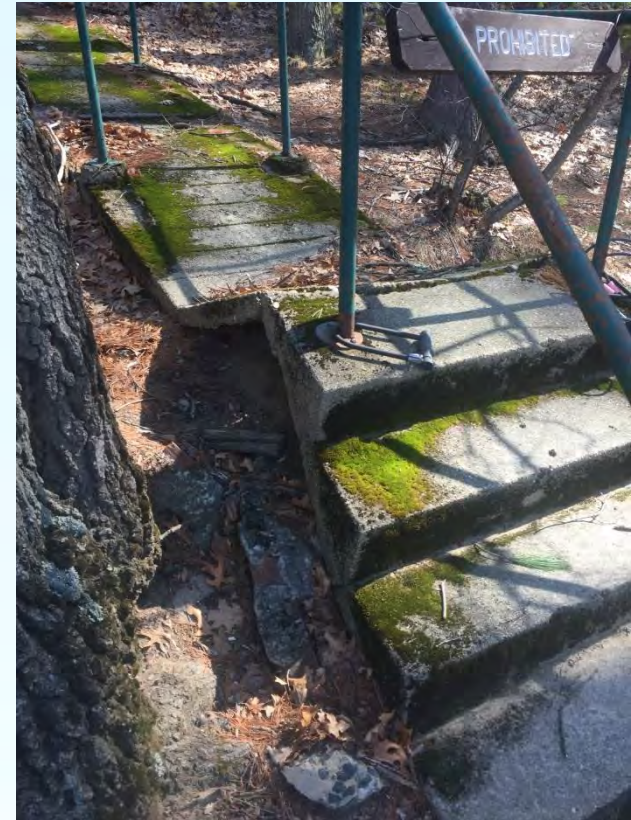
Existing stairs in an unusable state
