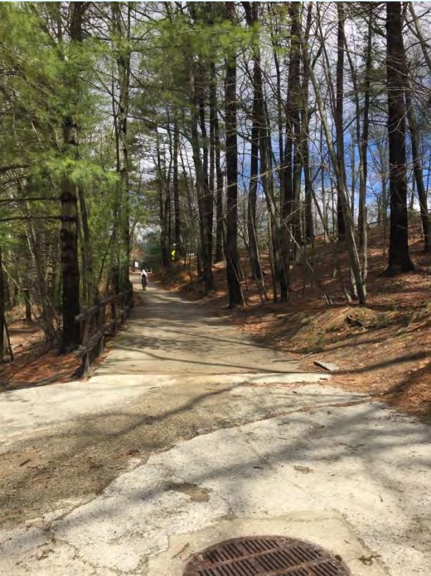
Erosion / runoff issues at the base of the existing E-Ramp
