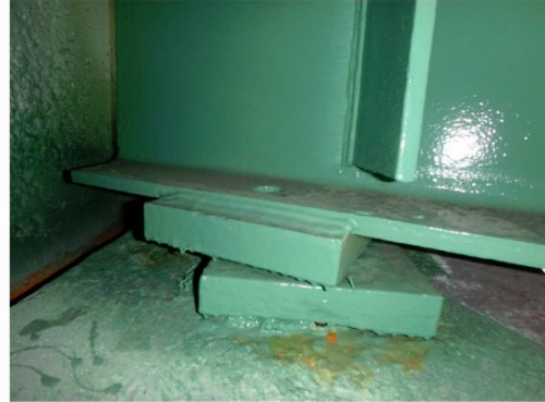
Photo 21: Span 4, Beam 31, West Abutment: Missing south anchor bolt and rotated bearing
