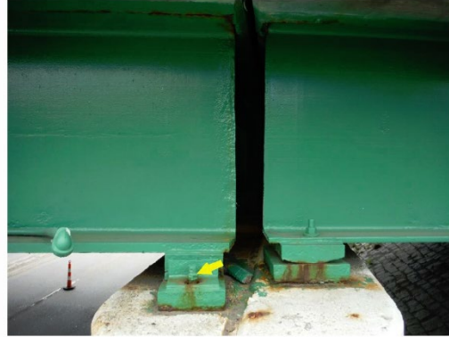
Photo 11: Heavy section loss to the anchor bolt nut of the Beam 37 bearing at Pier 2 in Span 5.
