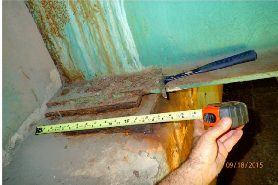
Photo 30: Typical bearing, over extended without anchor bolts.
