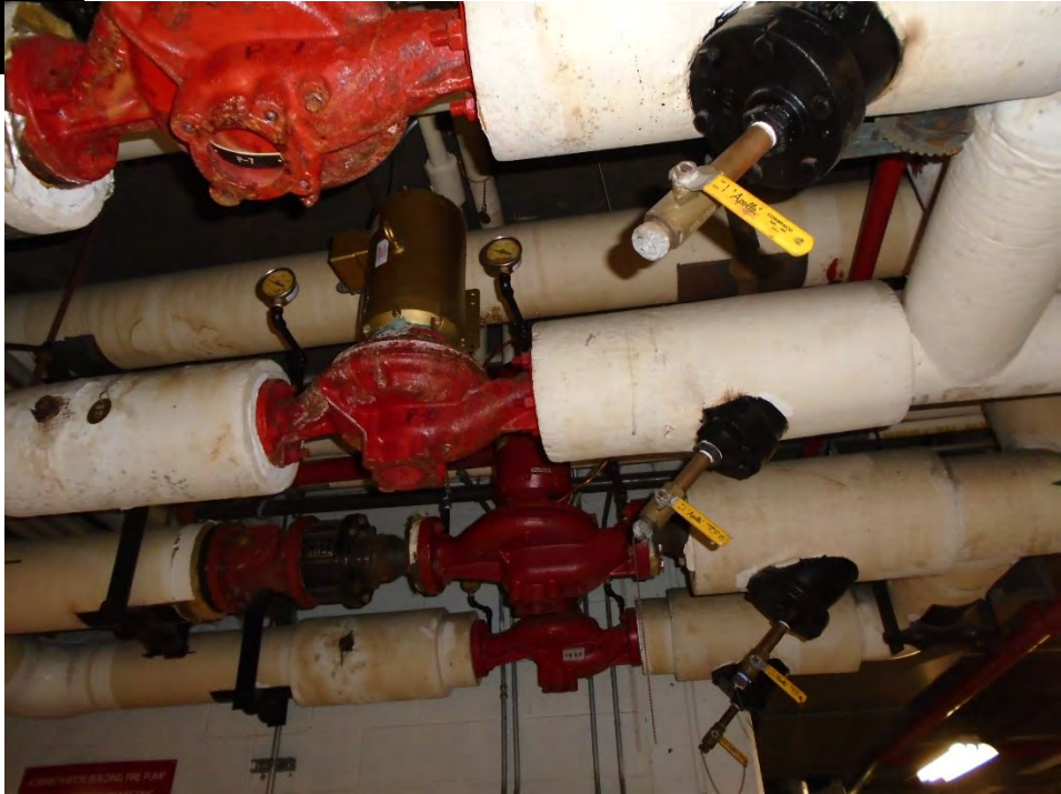
Photograph No. M-03 Heating water zone pumps
