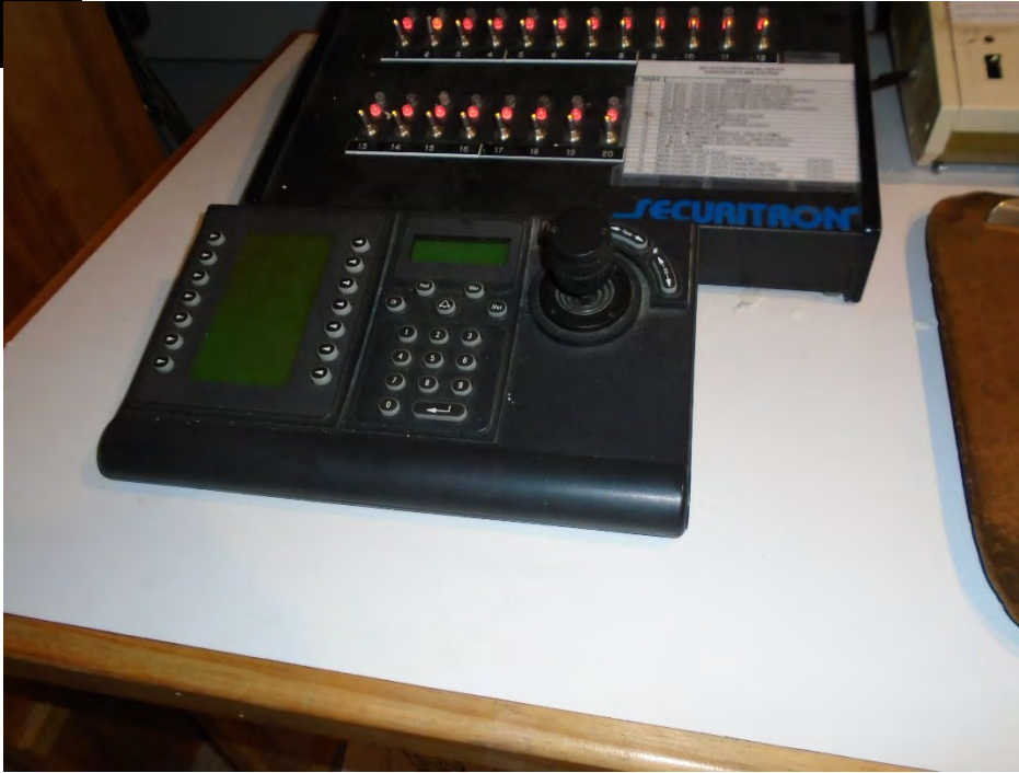
Photograph No. E-07
