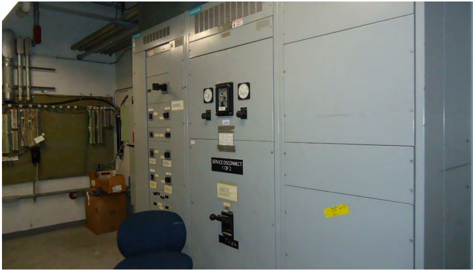
Photograph No. E-03
