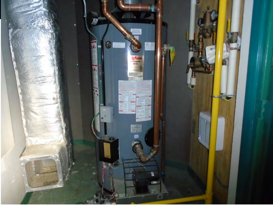
Photograph No. P-03 Typical modular housing domestic water heater
