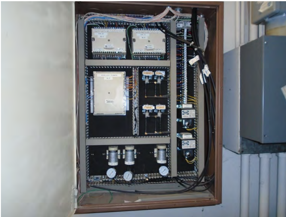
Photograph No. M-12 Hybrid Pneumatic / Digital HVAC system controls
