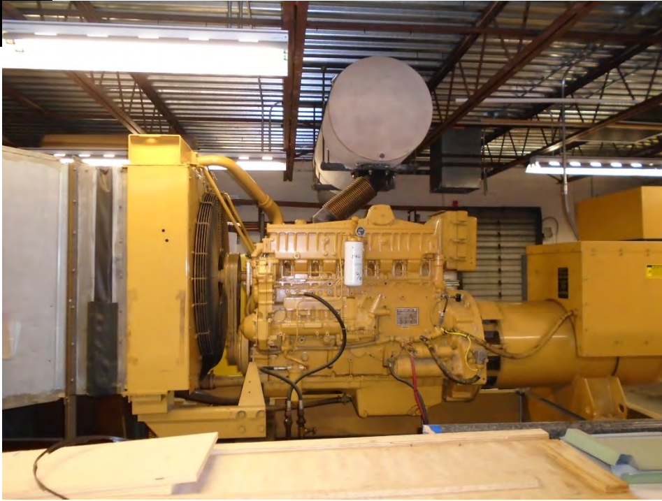
Photograph No. E-05 350-kilowatt diesel generator (Modular Housing, Visitor Building, Gate House, Morton)
