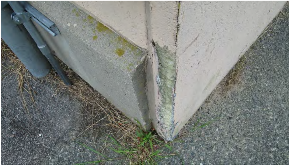
Photograph No. EX-2 Exposed insulation at Gate House exterior wall.
