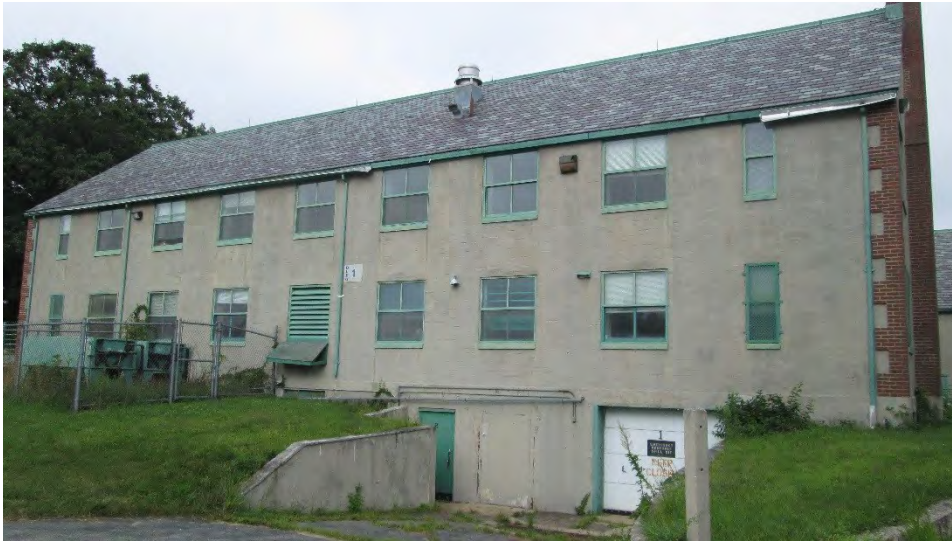
Photograph No. R-7 Missing gutter at Administration Building.
