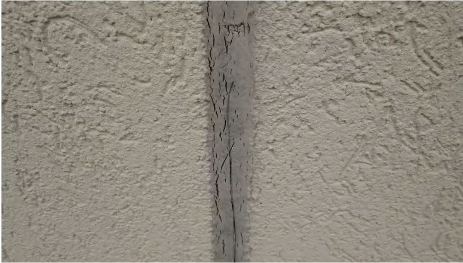
Photograph No. EX-6 Failed sealants at Visitor Building.
