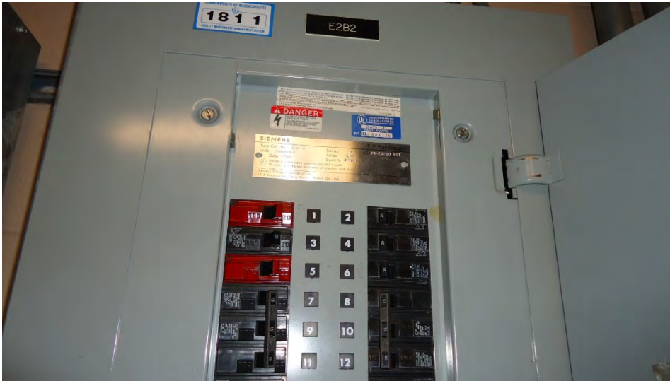
Photograph No. E-06 Typical Secondary Electrical Distribution Breaker Panel
