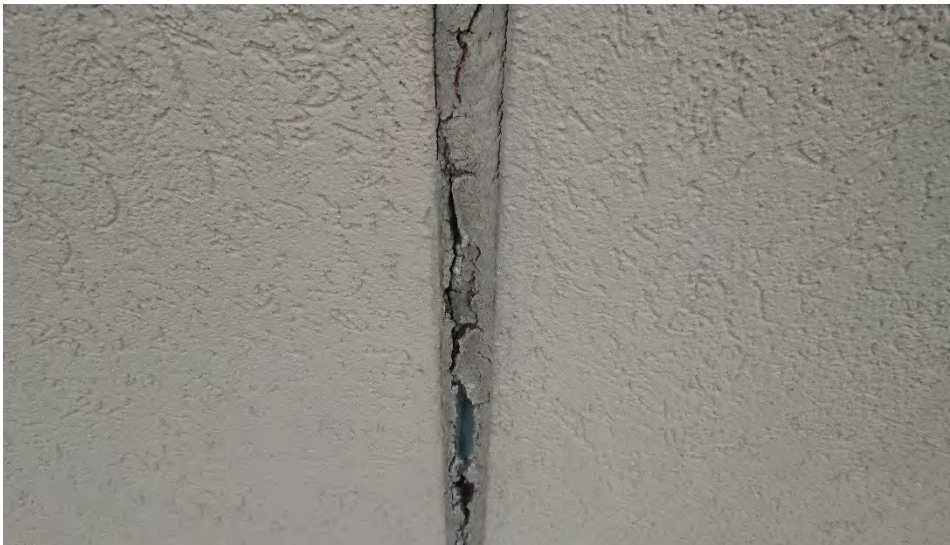
Photograph No. EX-3 Failed sealant at Gate House wall.
