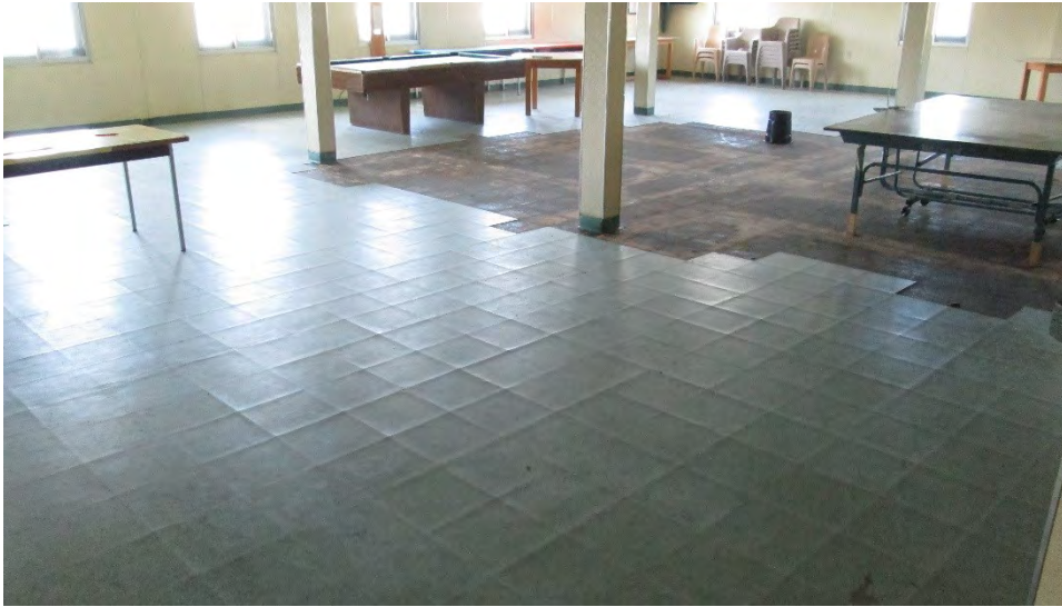
Photograph No. I-6 Failed flooring at Modular Housing, upper level.
