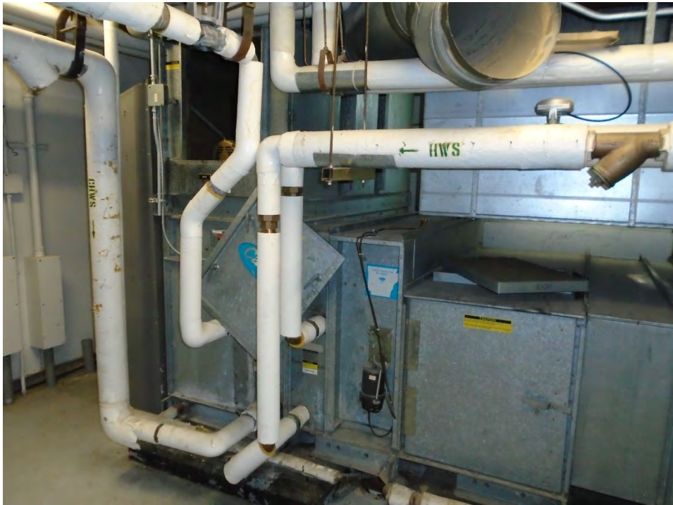
Photograph No. M-04 Central station air handling unit with chilled water coils serving the Administration office areas
