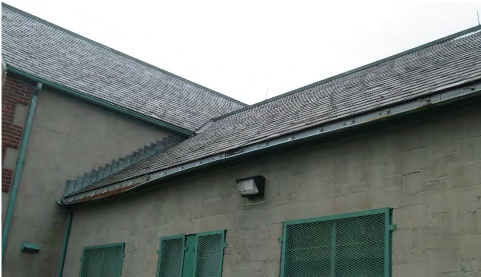
Photograph No. R-6 Failed gutter at Administration Building.
