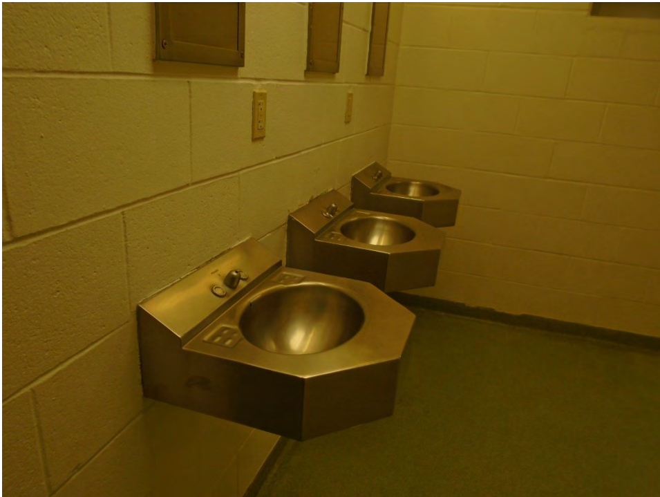
Photograph No. P-04 Typical correctional grad plumbing fixtures
