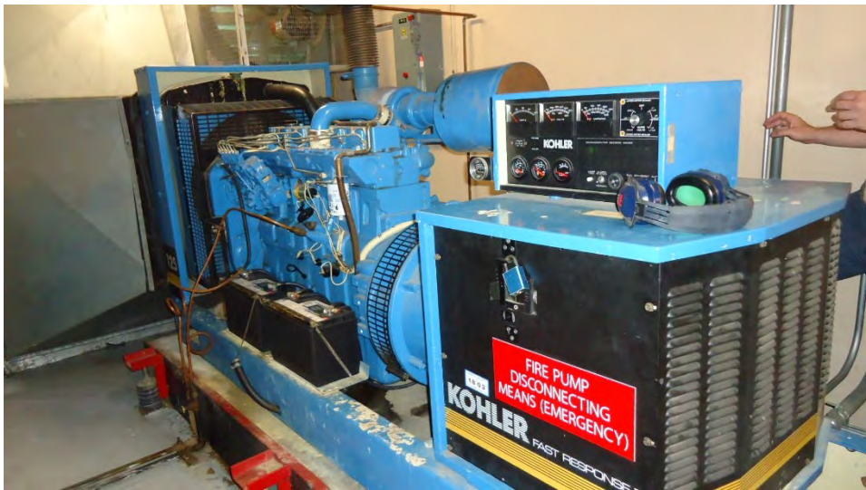
Photograph No. E-04
