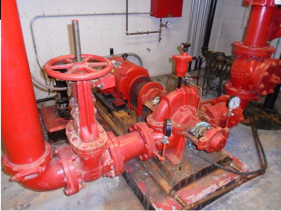
Photograph No. FLS-03 Electric fire pump
