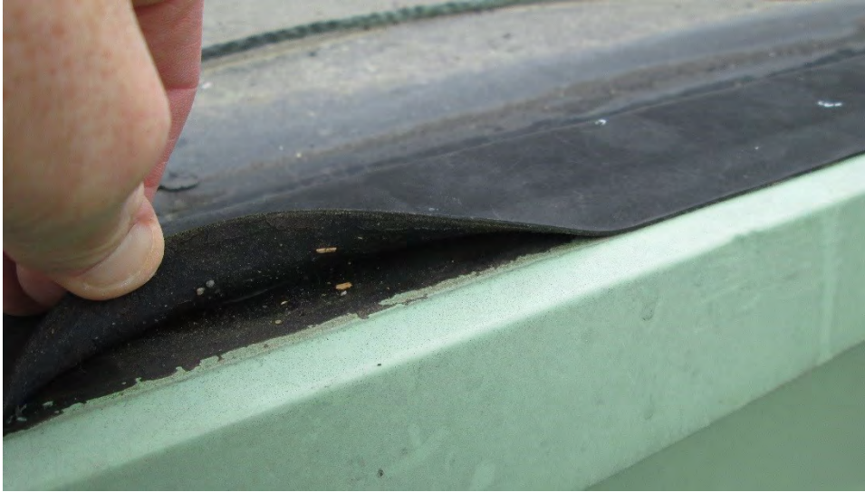
Photograph No. R-6 Poorly adhered flashing at Visitor Building roof.
