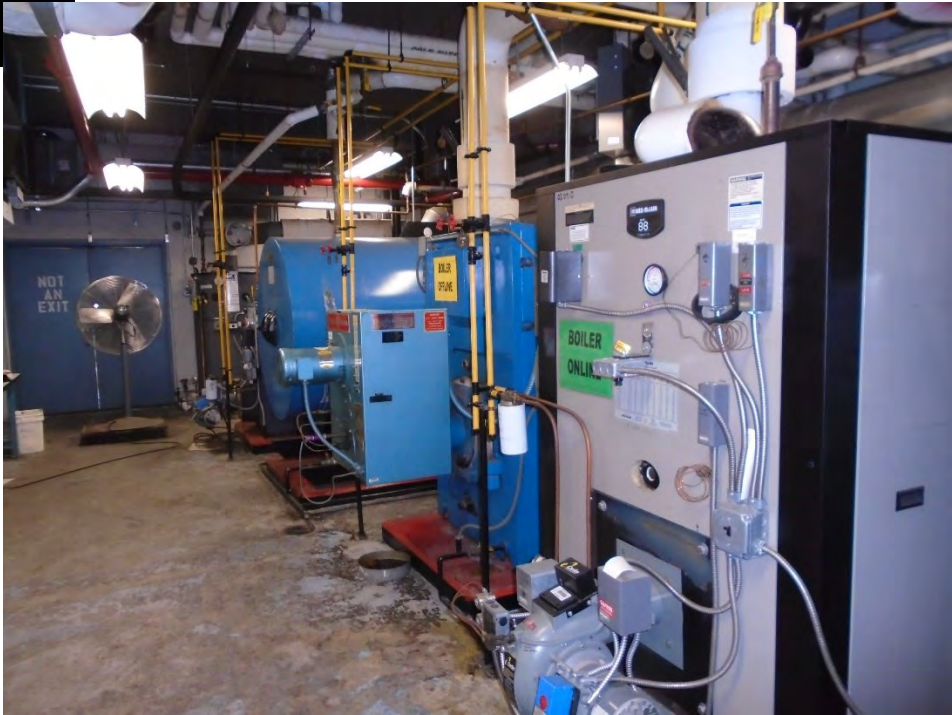
Photograph No. M-11 Heating water boilers
