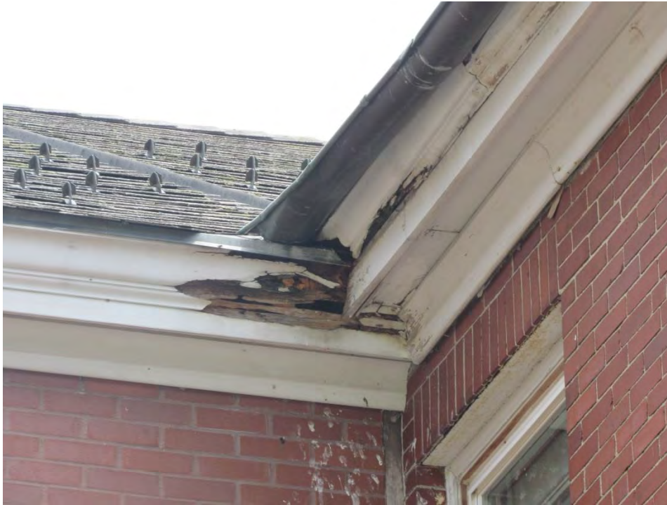
Photograph No. EX-5 Rotted Trim at Front Elevation of Main Building
