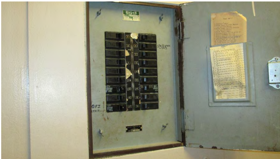
Photograph No. E-02 1939 Vintage Breaker Panel
