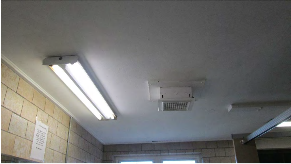
Photograph No. E-03 T-12 Fluorescent Lighting
