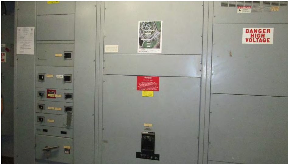
Photograph No. E-01 Primary Electrical Service
