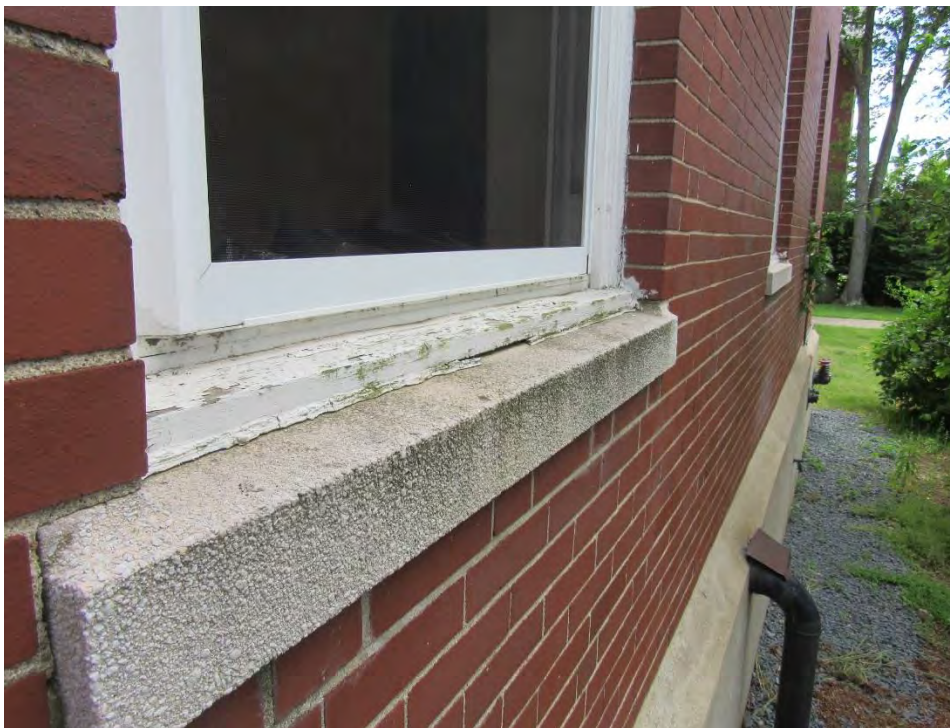
Photograph No. EX-6 Rotted Window Frame at Front Elevation of Main Building
