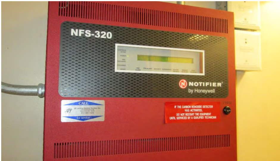
Photograph No. FLS-01 New Fire Alarm Control Panel
