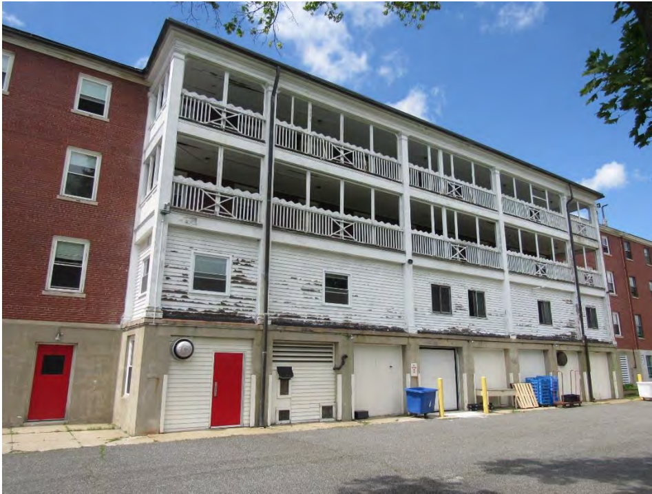
Photograph No. EX-9 Deteriorated Balcony at Rear Elevation of Main Building
