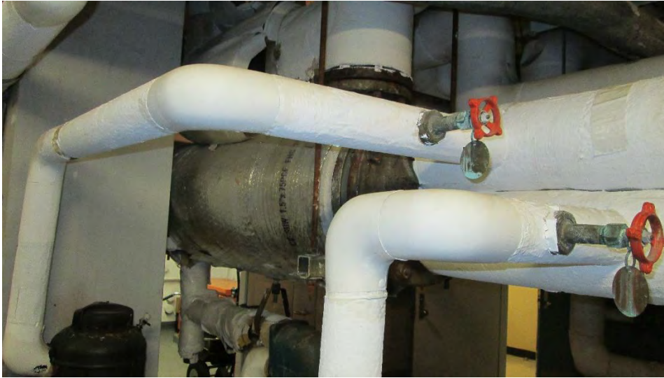
Photograph No. M-01 Shell and Tube Heating Water Converter
