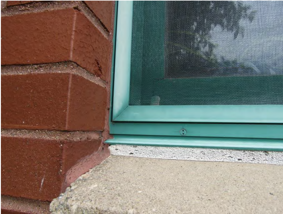
Photograph No. EX-1 Failed Window Perimeter Sealants at Main Building Roof
