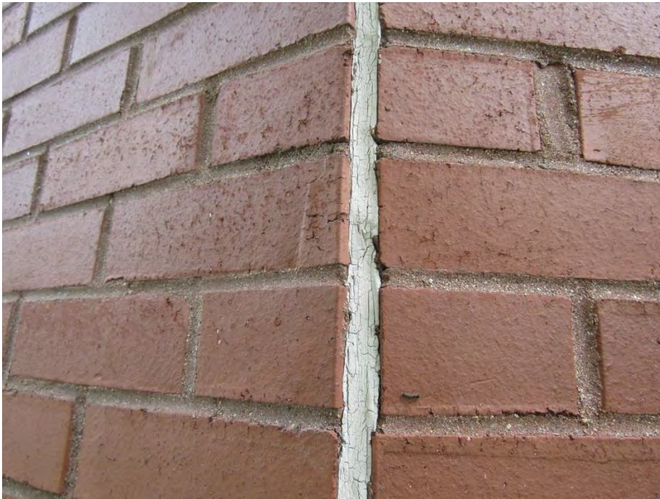
Photograph No. EX-2 Failed Control Joint Sealant at Main Building Exterior Wall
