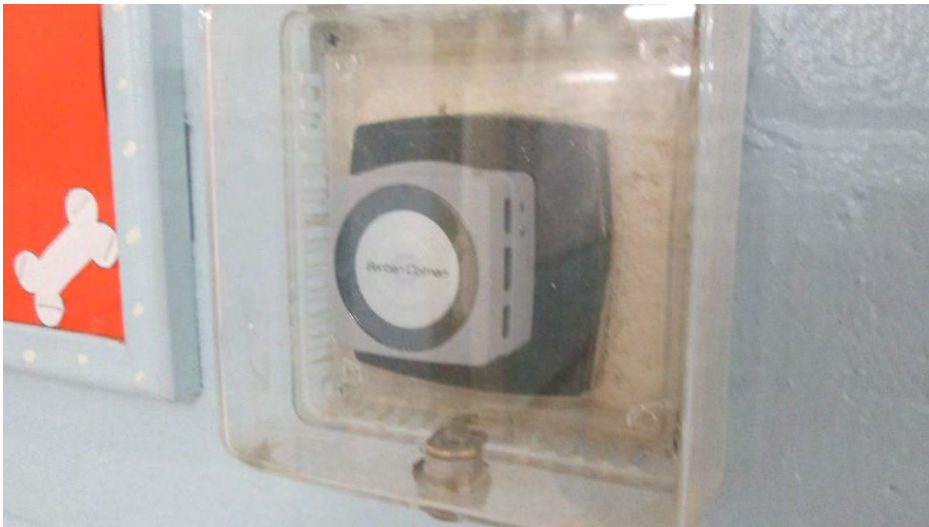
Photograph No. M-08 Pneumatic Controls
