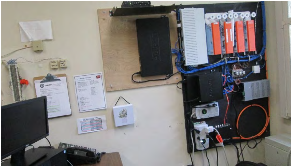
Photograph No. E-05
