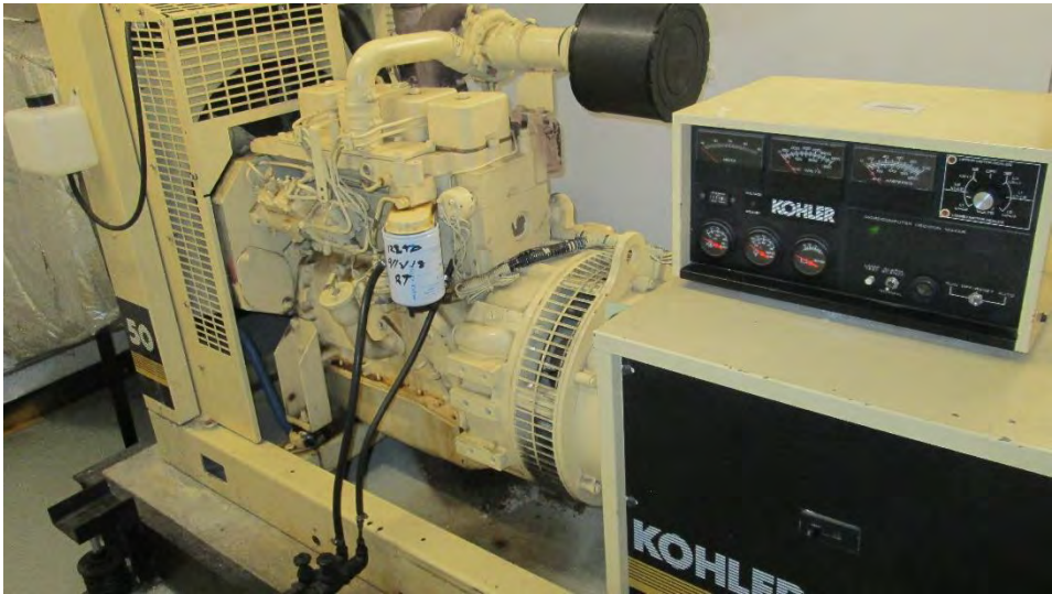
Photograph No. E-04 50 Kilowatt Emergency Power Generator
