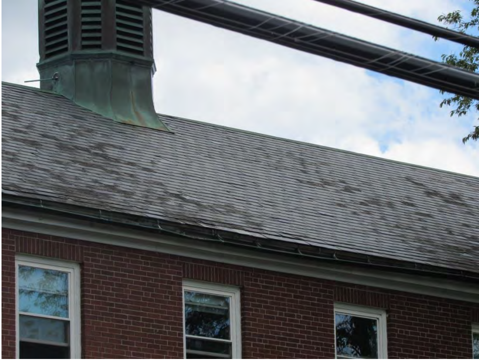
Photograph No. R-7 Surface Scaling at Main Building Roof Tiles
