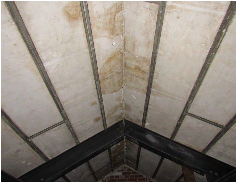
Photograph No. R-1 Water Stains at Underside of Main Building Roof
