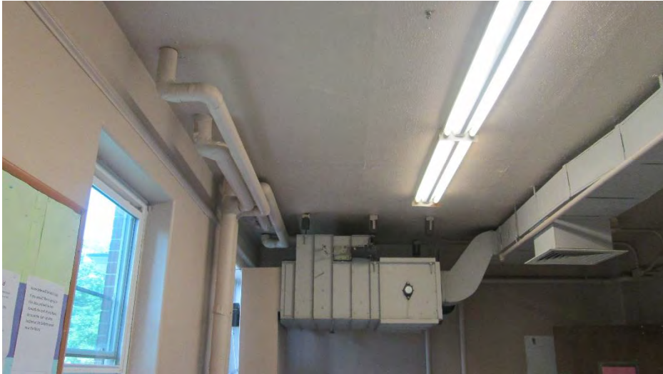
Photograph No. M-07 Laundry Room Heating and Ventilating Unit
