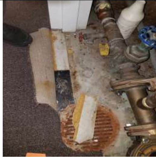
Kindred floor tile/mastic under carpet, asbestos
