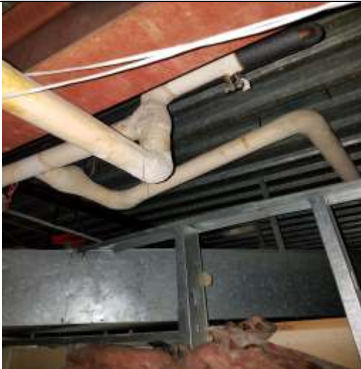
Asbestos pipe fittings in cafeteria plenum
