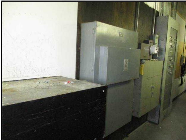
Main electrical service.
