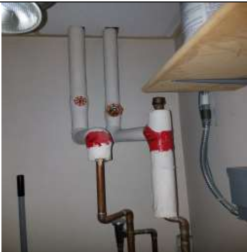
Janitor closet 2071, asbestos pipe fittings
