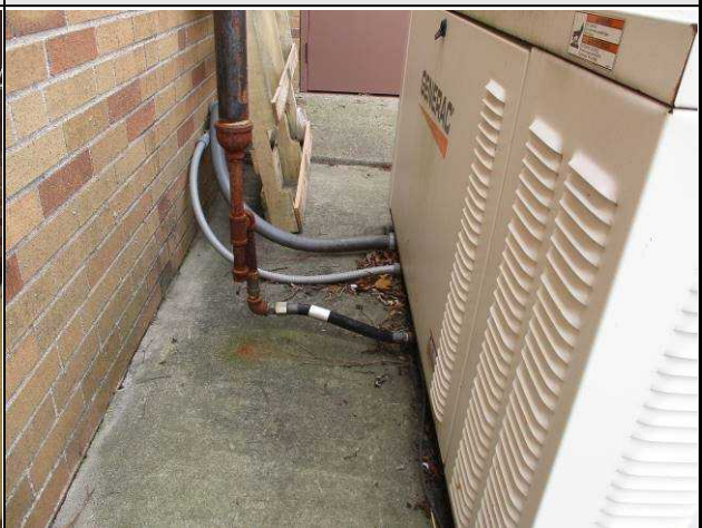
Natural gas piping to the emergency generator.
