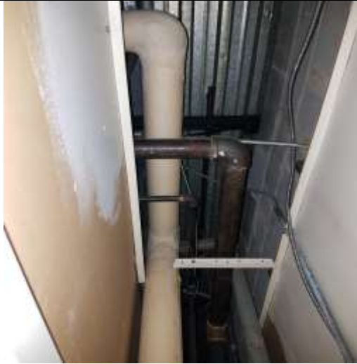
Kindred space, asbestos fitting
