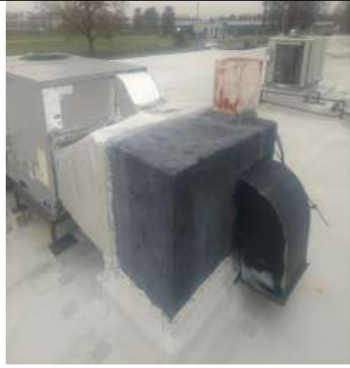
Tar mop on duct, asbestos
