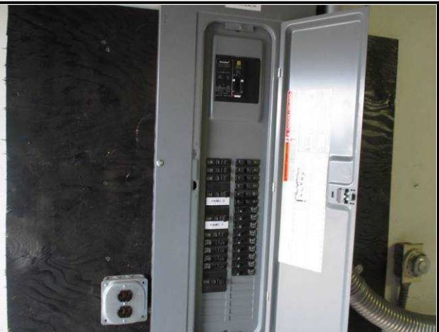
Typical electrical panel.
