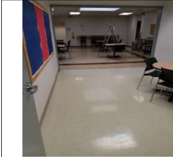
Newer floor tile in cafeteria
