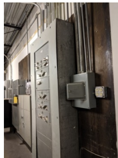
Limited electrical room serves all mechanical needs.
