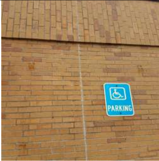
Wall expansion, not asbestos
