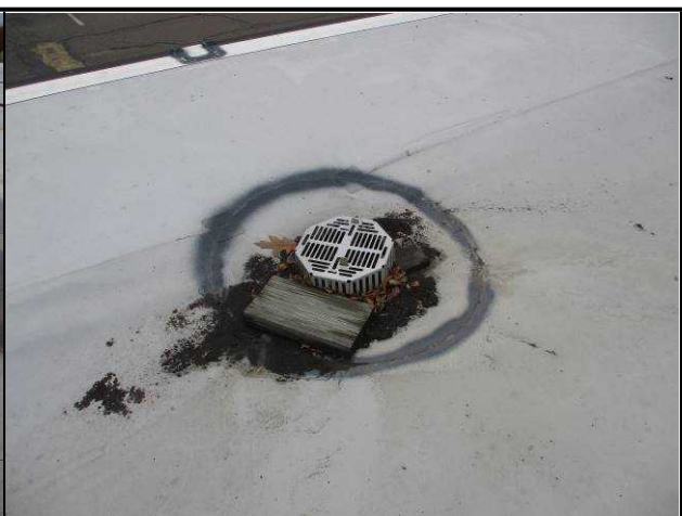
Several of the roof drains were found to be clogged with debris.
