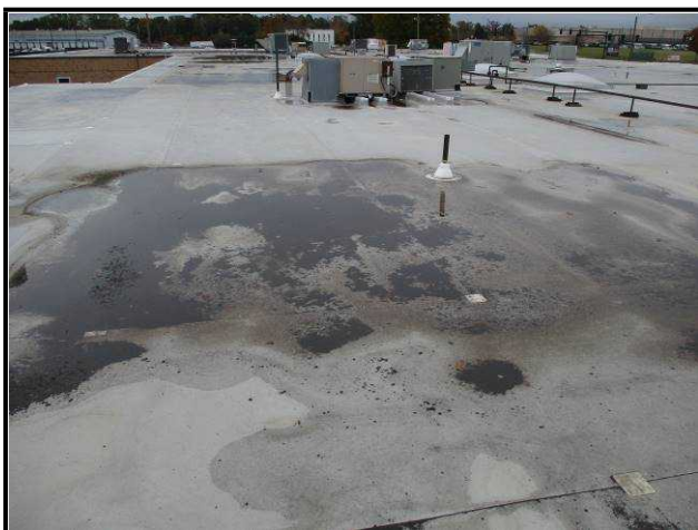
Severe ponding was observed throughout the roof area.
