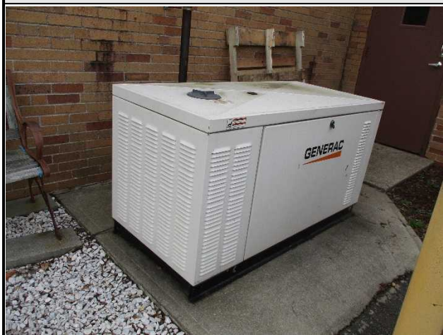
Emergency generator condition.
