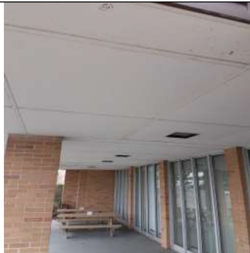
Asbestos ceiling panels at rear entrance
