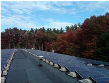
Solar Array on the roof of Delaware Valley's Tewksbury facility
