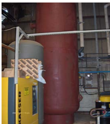
3,000 gallon vertical receiver
