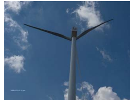
Wind Turbine Generator
