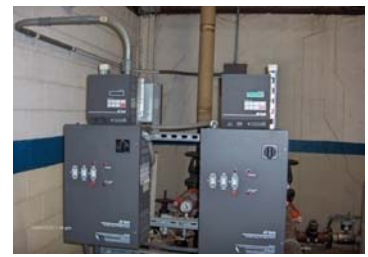
Plant Booster Pump
