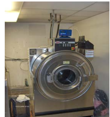
The replacement washing machine installed by Marriott
