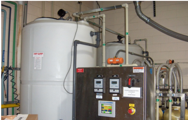
System for reusing water from container washing operations at Rohm & Haas (Dow), Marlborough
