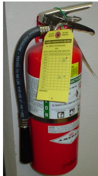
A portable fire extinguisher with a maintenance tag
