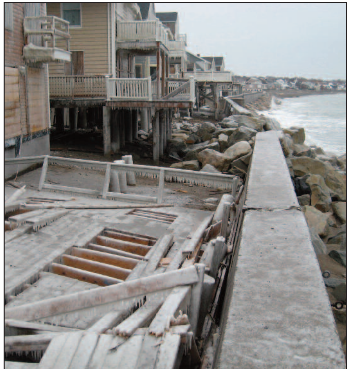
Decks, stairs, siding, and other parts of these buildings were damaged by waves and flooding in a northeaster. Repairs to these houses will require permits under the State Building Code and Wetlands Protection Act regulations, and possibly the local wetlands bylaw.
