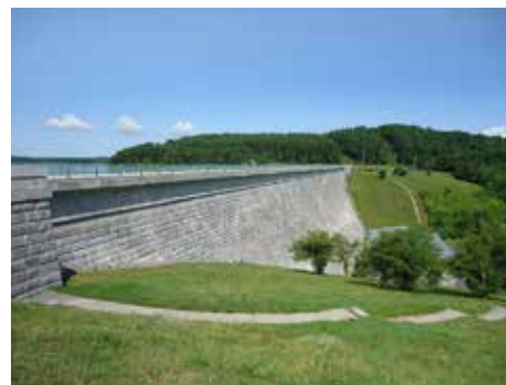
The Wachusett Dam is designed to impound up to 65 billion gallons of water.
