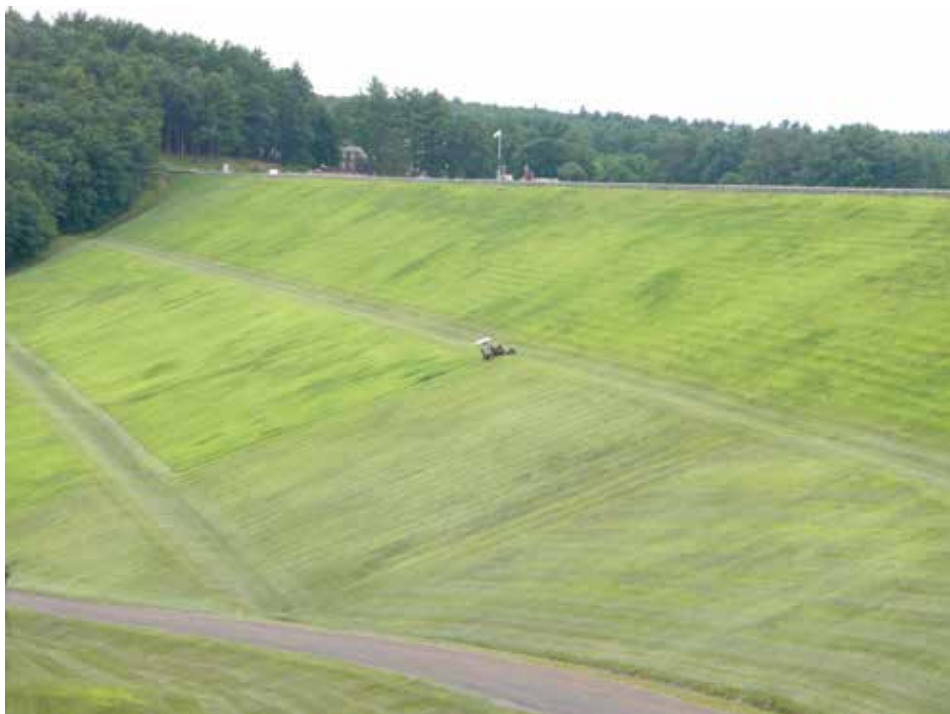
A slippery slope? This view of the back of Quabbin Reservoir's Winsor Dam shows the daunting task facing the mower (in the center of the picture). It takes two days to mow the whole face of the dam.
