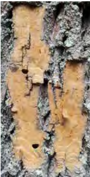
This picture details the bark damage caused by feeding EAB larvae. Note the 'D'-shaped exit hole made by the mature EAB, which kills upper branches of the tree and leaves it vulnerable to disease.
