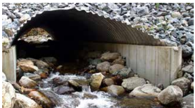
Following Tropical Storm Irene, the Green Mountain National Forest found that culverts recently replaced using Stream Simulation Design, on which the Stream Crossing Standards are based, suffered little damage and safely passed huge volumes of water, gravel, and debris that clogged and destroyed other traditional culverts in the area. (U.S. Forest Service photo)
