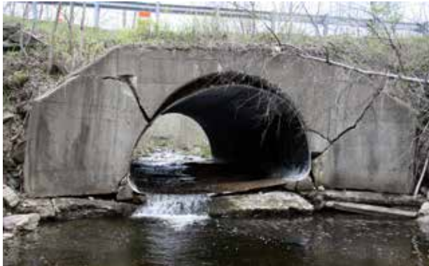
Crossing failure leads to road closure. (Westfield River Wild & Scenic Committee)
