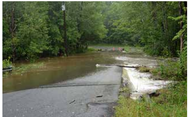
Streams move water, debris, and sediment. Crossings should be designed to accommodate transport of these materials, otherwise they may become clogged or overtop during severe rain events. (Carl Lafreniere photo)
