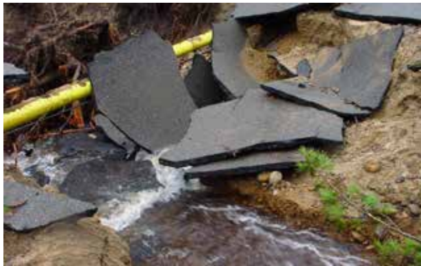
With an increase in the number and intensity of extreme storm events, local public work departments are reporting an increase in road failures and closures due to overwhelmed culverts. (Unknown photo)
