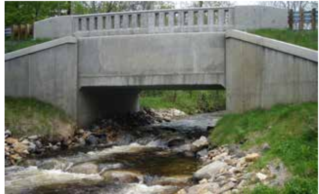
This prefabricated bridge design restored passage for vehicles, as well as fish and wildlife. (Westfield River Wild & Scenic Committee)
